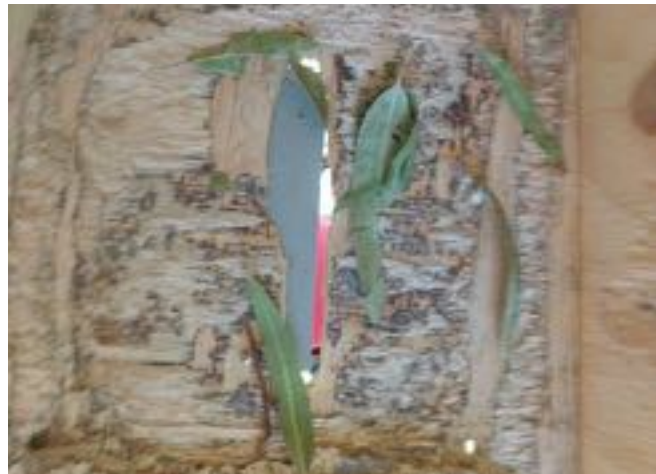
Figure 16: Damaged Possum Box, Windsor St South, replaced with a sacrificial floor.
