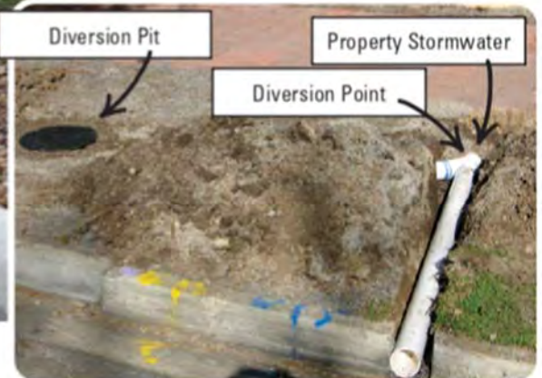
Stormwater diversion pits capture rain water from property overflow and store the water in a pit slowly dispersing into the nature strip supporting tree growth.
