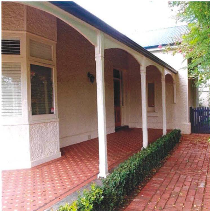
Western verandah. The current owners laid replica ceramic tiles to replace the damaged verandah floor.
