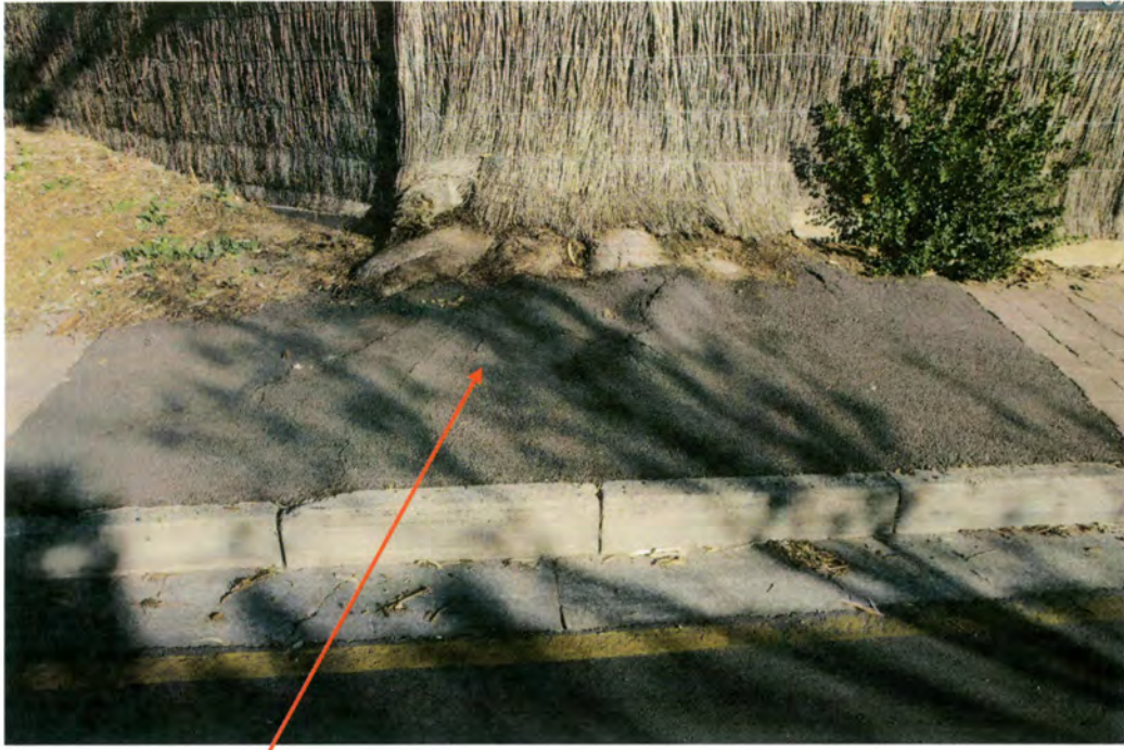
Cracking and lifting creating the hazardous condition
