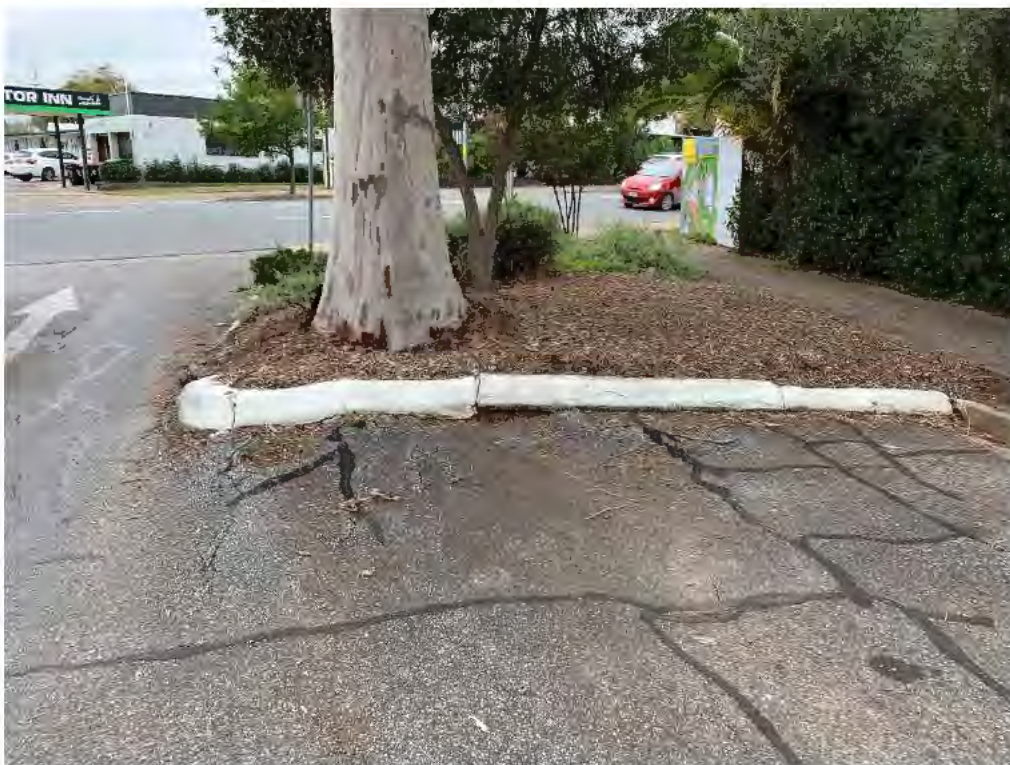
Photo 3: showing disruption of bitumen surface by tree roots.
