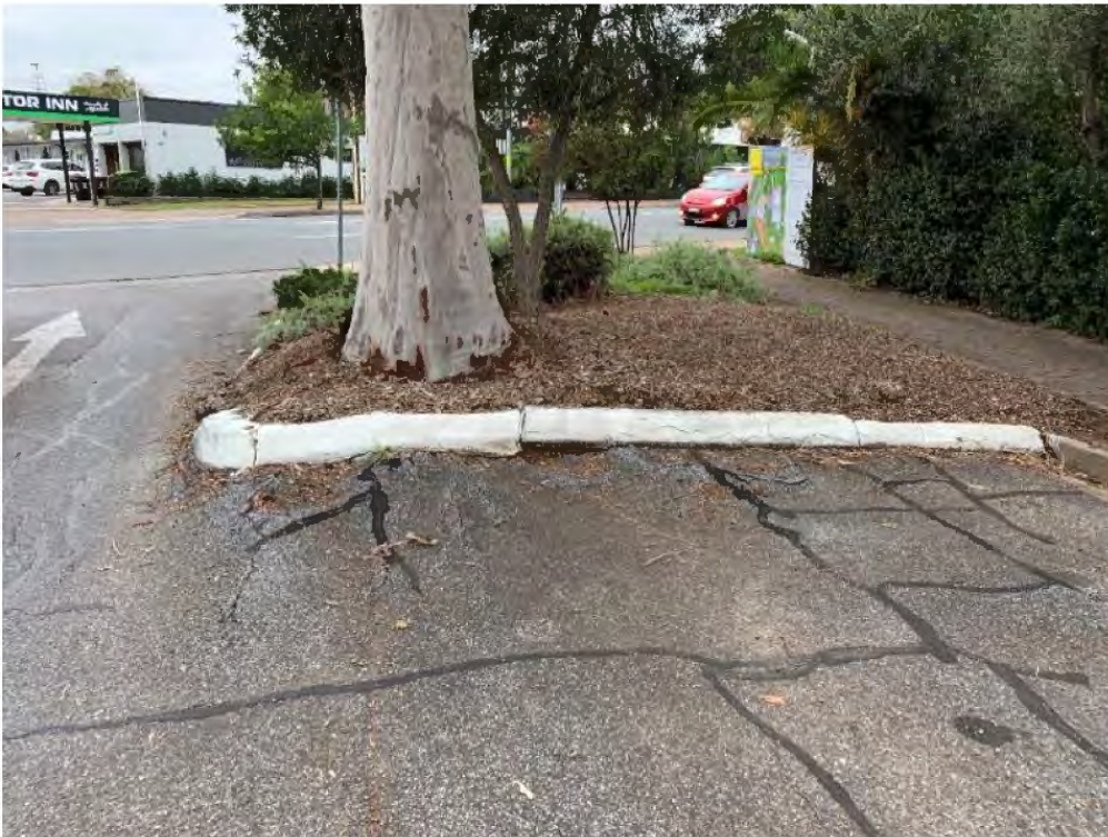
Photo 1: showing disruption of bitumen surface by tree roots.
