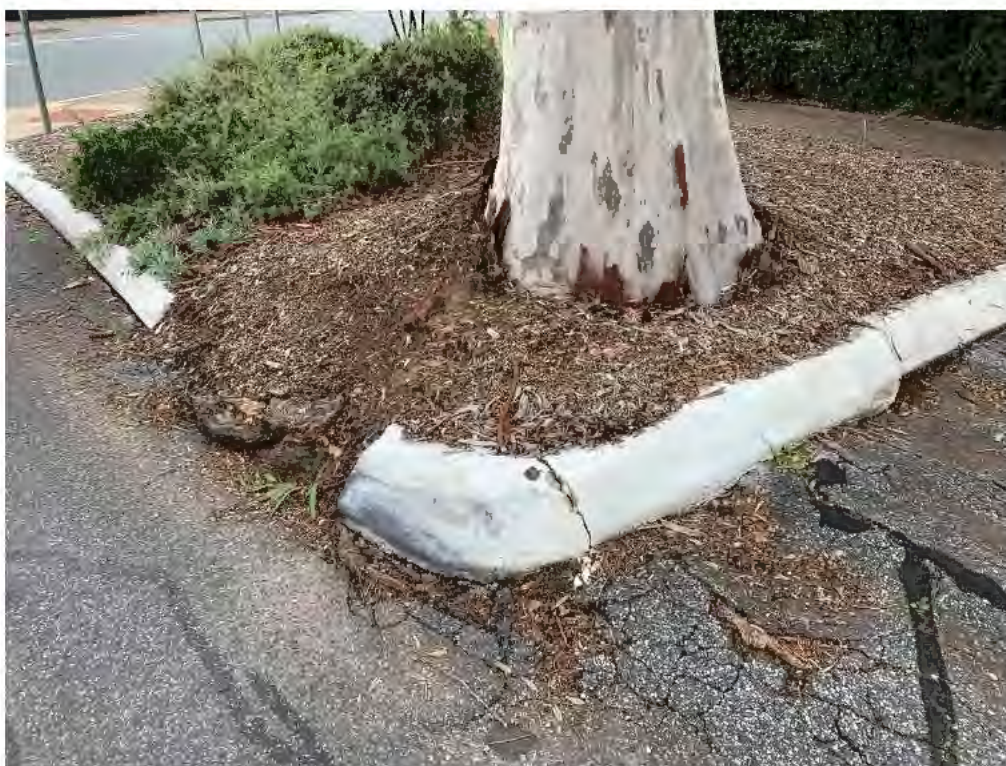
Photo1: showing kerb disruption at tree base.
