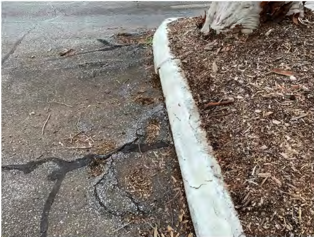
Photo2: showing kerb disruption at tree base.
