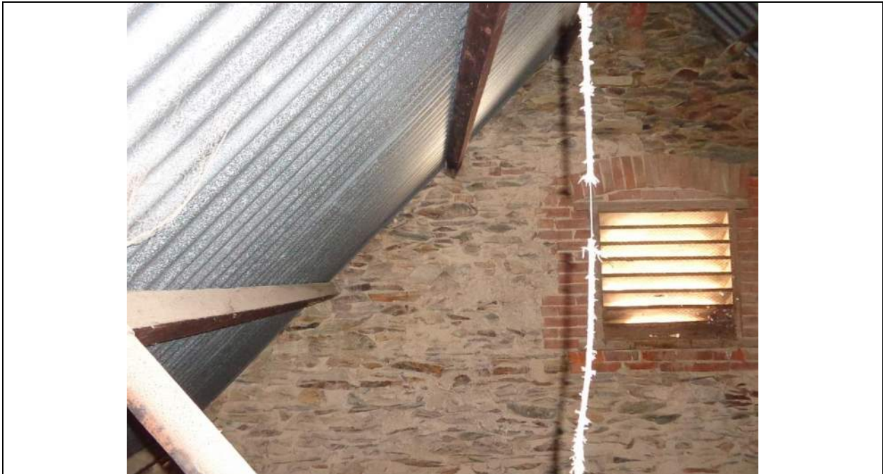
PHOTO 47 – A view of the stone masonry gable end to the eastern end of the roof looking south. The purlins are pocketed into the stonework once again which can be problematic as noted earlier.
