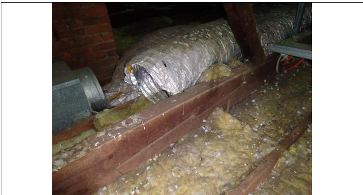
PHOTO 4 – The main roof trusses are a substantial span (approximately 19100mm) and have been constructed with a bottom chord splice with a metal plate to the top and bottom face of the bottom chord member and two bolts. The splice joints looked in reasonable condition and splitting or joint slip was not evident although it would seem that some truss ‘sag’ has occurred over the years.
