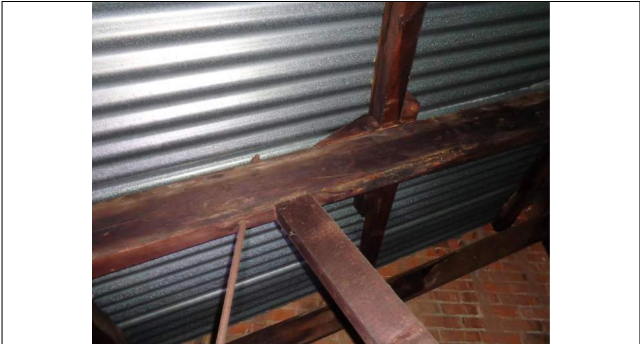
PHOTO 5 – Typical top chord web joint which is a mortise and tenon joint with adjacent tension tie rod. The purlins have no specific tie down other than skew nails and anti-slip blocks. The purlins are regularly ‘scarf cut’ and joined over the top chord members. The roof sheeting appears in a satisfactory condition from beneath generally speaking.
