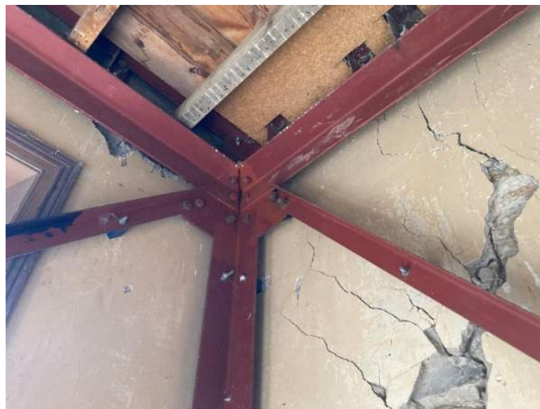
Figure 8 – Cracking to Central Tower
