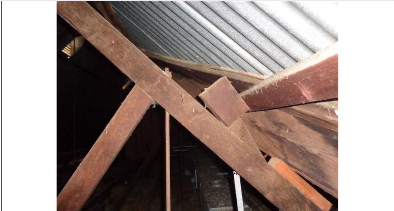
PHOTO 27 – Some of the purlins have been poorly supported around the hip valley rafter, extra blocking has been included at a later date possibly due to excessive truss sag and some blocks are rotating off of their support as seen above.
