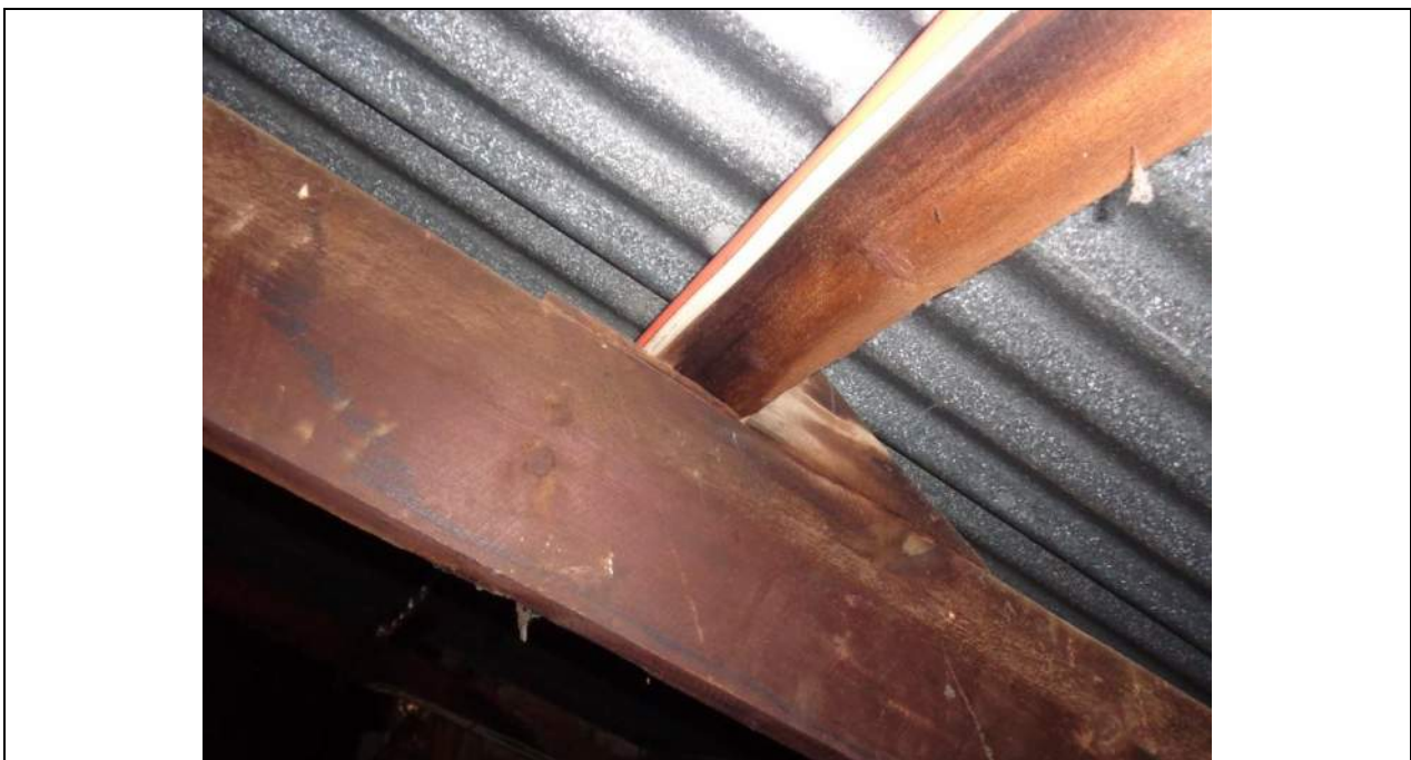
PHOTO 6 – Another view of a purlin; however, this purlin has been packed off of the top chord. This detail has been repeated in numerous locations. This may have to do with the original truss fabrication, to try and obtain a level roof plane or it could be a later inclusion if the trusses have deflected more over time. Some of the purlin and top chord gaps are significant.
