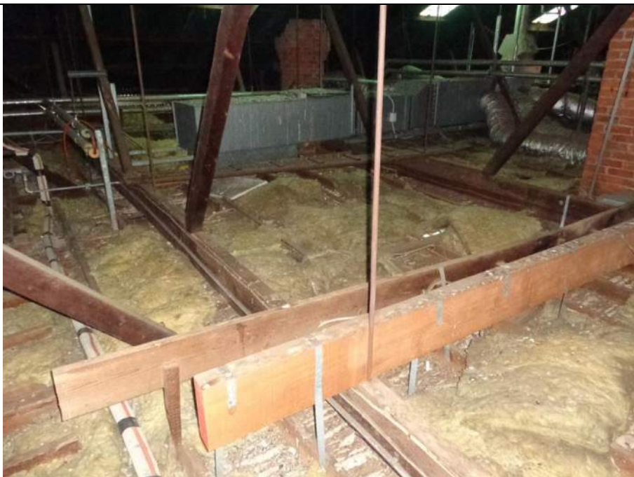
PHOTO 24 – Newer and older hanging beams. Metal tension straps have been used for the newer hanging beam rather than timber soldiers. Note the excessive deflection in the original hanging beam. The plaster lathe ceiling and timber battens are evident in the foreground but there is additional ceiling lining below this level which has also added additional loads to the trusses.
