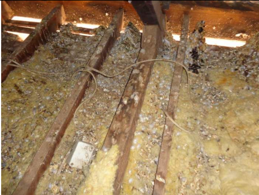
PHOTO 45 – As per photograph 44 comments above. The pigeon and rat infestation has ruined the insulation which will need to be discarded and replaced once the roof space is made secure again.
