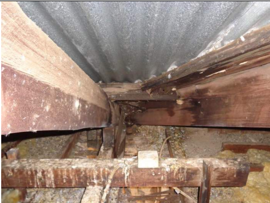
PHOTO 26 – The hip valley rafter appeared to have suffered some rot to the end. The eaves were open at this location and the pigeons can freely enter and have made a significant and unhealthy mess. Where pigeon excrement has been allowed to accumulate the roof sheeting is showing greater signs of corrosion/deterioration. Water damage/staining was also evident in some locations.
