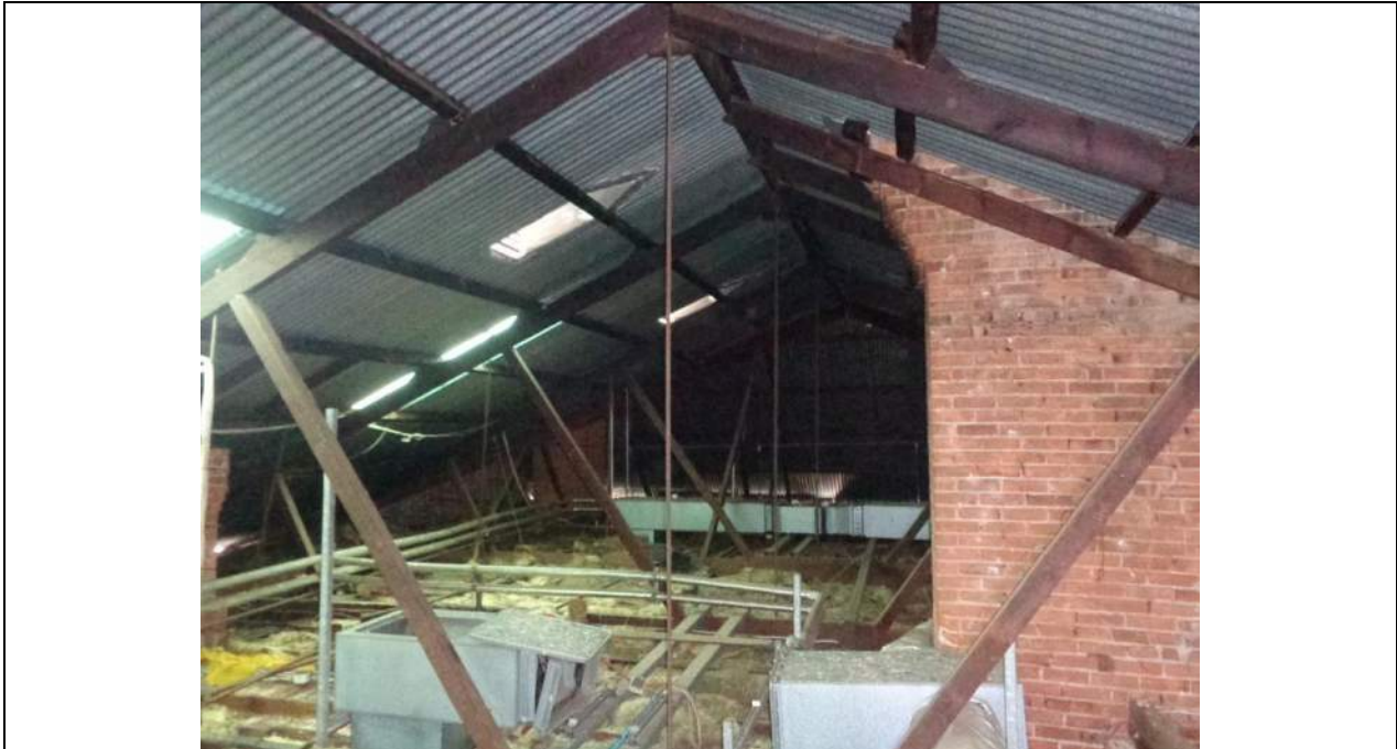
PHOTO 1 – General view of the roof space from the centre looking west. The main trusses can be seen and infill rafters around the brick chimney penetration. The main trusses are fabricated with Douglas Fir (Oregon) timber of reasonable grade and metal tie rods. The purlins are also Oregon and vary in size depending on the truss spacings. Intermediate ceiling joists and hanging beams have also been adopted.
