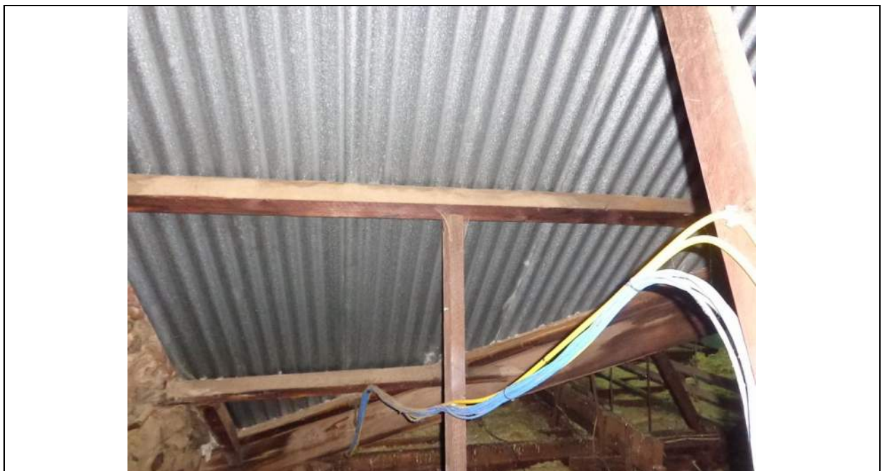
PHOTO 52 – As per photograph 51 another propped purlin. It is unclear why these purlins are propped when adjacent purlins are doing a full span.
