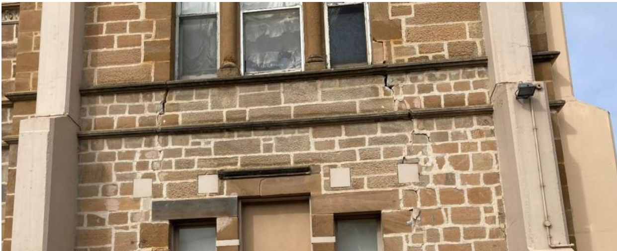
Figure 14 – Comparison of Cracking at NW Corner of Western Wing (2021 photo below and 2011 photo above)
