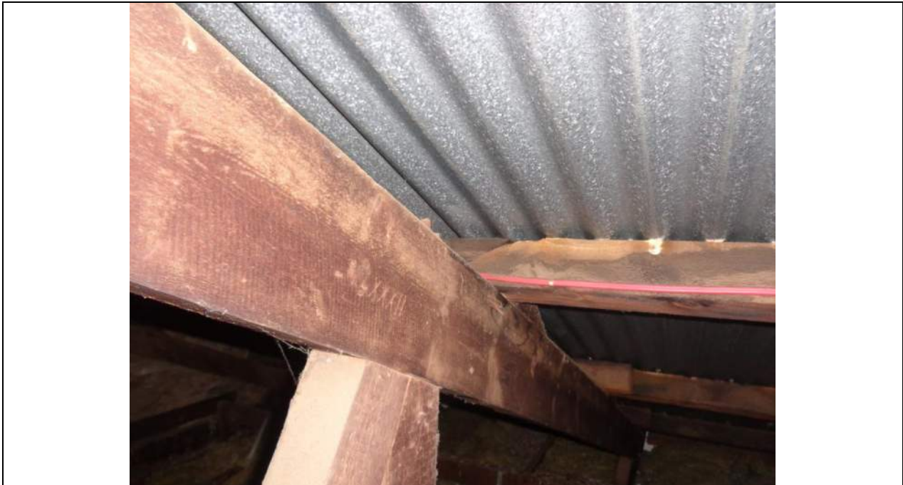
PHOTO 7 – Typical truss joint with a vertical web included to provide an internal support point over a common internal masonry wall. Note the Roman numerals stamped into the top chord which corresponded with the webs indicating that the trusses may have been made on the ground, marked, and reassembled on top of the walls. Note also the ‘scarf cut’ to the purlin member.
