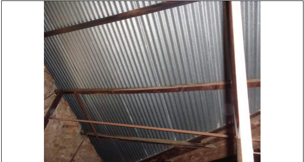
PHOTO 67 – Northern gable to the western end of the roof. Note the excessive deflection in the roof purlin.
