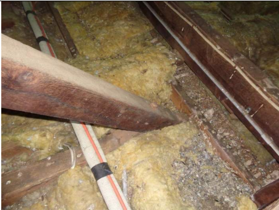
PHOTO 23 – Typical truss top chord with a single bolt through the top and bottom chord members. There is a small heel block present in the joint. It appears as if there is a load bearing masonry wall located below the pitching line of these trusses.
