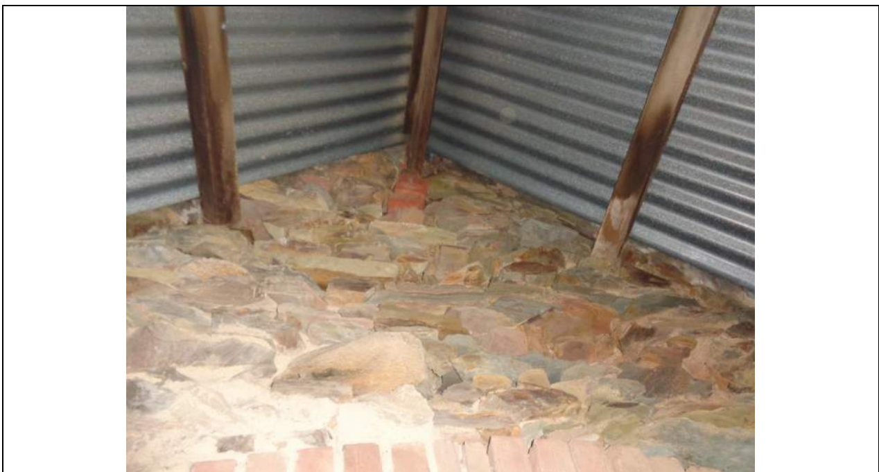
PHOTO 48 – As per photograph 47. The mortar has deteriorated significantly to the upper peak of the gable (difficult to get a full appreciation from the photograph) and will need some attention/rectification.
