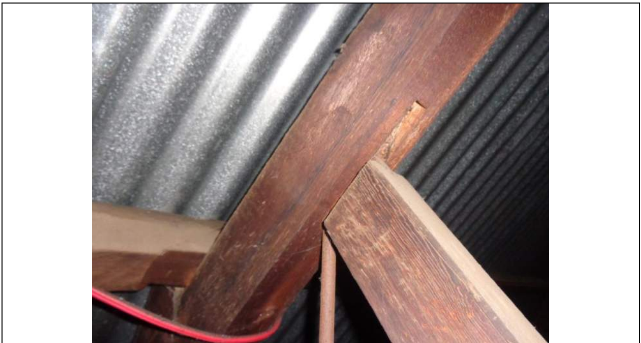
PHOTO 40 – As per photograph 39 another view of the mortise and tenon joint. The purlin also appears to be notched (original?).
