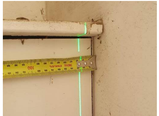
Figure 22 – Bowing of Wall at NW Corner of Western Wing
