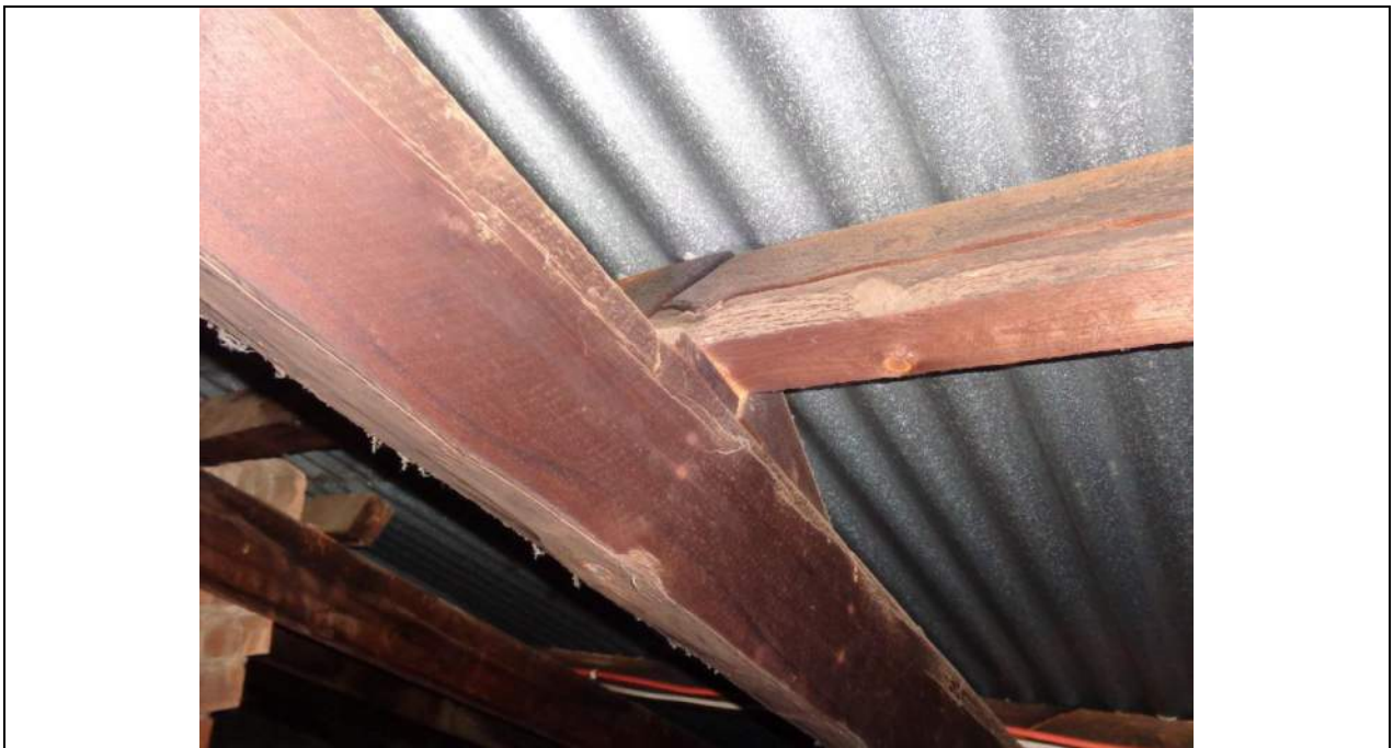
PHOTO 18 – The purlin has a drying ‘check’ which has caused a significant split and may be compromising the structural capacity. The purlin is also packed up quite significantly from the top chord. The truss top chord has a number of drying ‘checks’ some visible to the bottom edge and passing up through the depth of the member which is more unusual.
