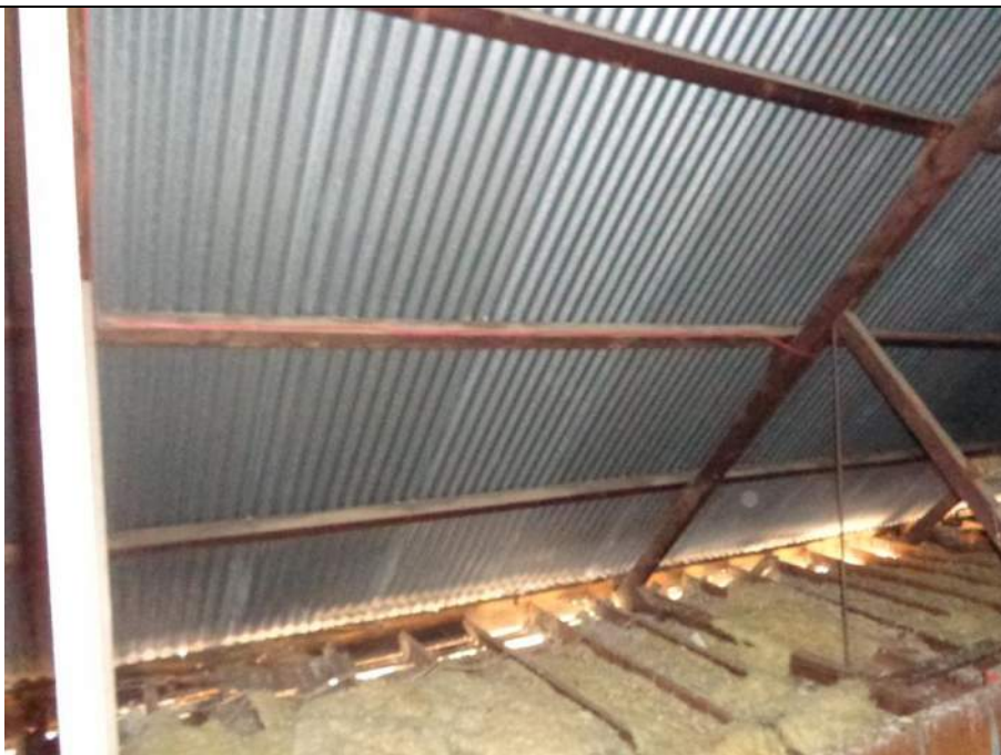
PHOTO 34 – Note the vented eaves to the eastern end of the building which have deteriorated significantly allowing pigeons to enter in multiple spots.
