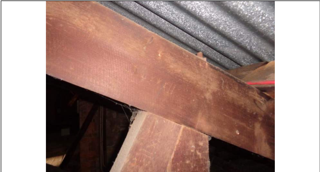
PHOTO 9 – As per photographs 7 and 8. The truss joint is still tight and in reasonable condition.
