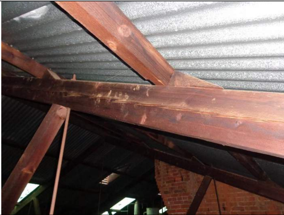
PHOTO 25 – A significant drying ‘check’ to the truss top chord. Some purlins appeared to sit up off of the top chord.
