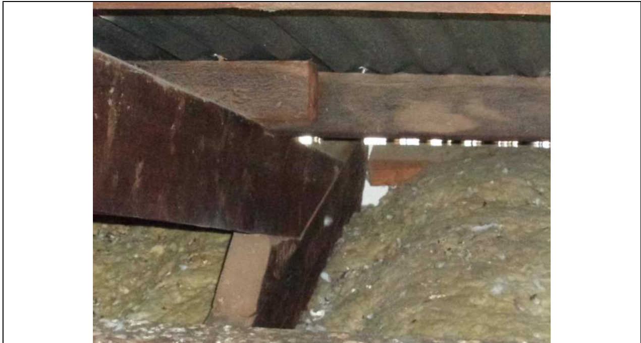
PHOTO 13 – As per photographs 11 and 12 showing the truss heel joint with heel block. The eaves are vented via timber battens. In numerous locations the battens are missing, and pigeons have nested prolifically in the roof space along with rats who tend to go after the pigeon eggs. The roof space is very messy and would be considered a health hazard to humans.
