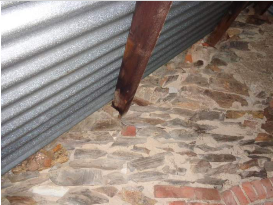
PHOTO 29 – Purlins pocketed into stonework gable end. It is unclear how far the purlins are embedded or their end condition. Sometimes purlins embedded into old stonework masonry can suffer water damage and consequent rot to their ends.
