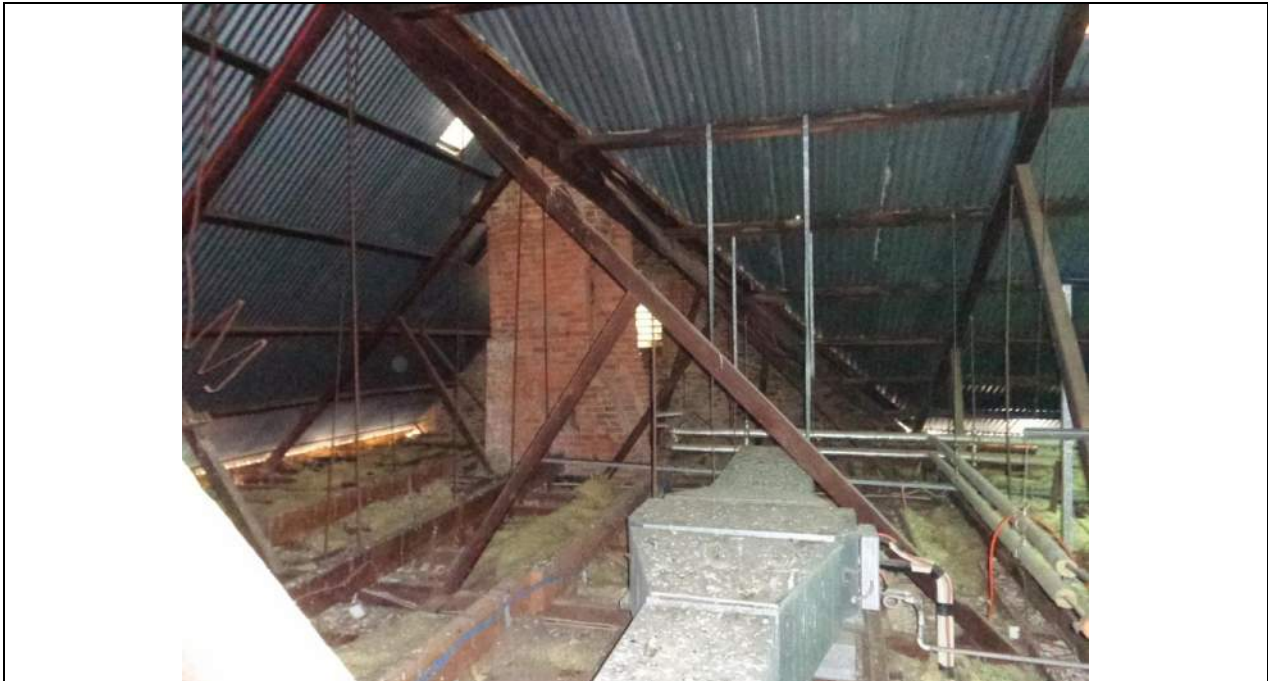
PHOTO 21 – A view of the eastern end of the roof. Note another chimney that may require some added lateral/earthquake restraint. Note some of the dip in the purlins, particularly when supporting suspended a/c ductwork. The extent of unrestrained top chords can be seen more readily in this photograph. Two newer rows of hanging beams have been added to the top of the truss bottom chord.
