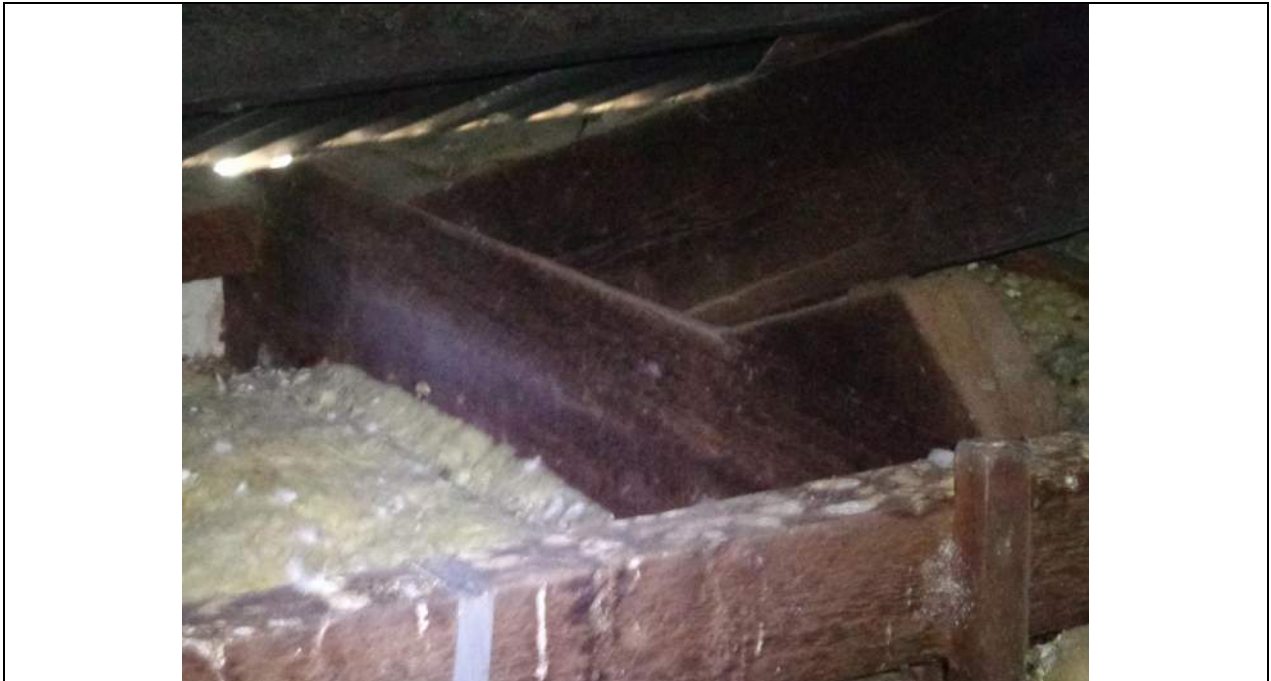
PHOTO 11 – Typical heel joint of the main span truss showing the bottom chord extending through to the back of the fascia beam and a ‘heel block’ (wedge) between the top and bottom chord with a single bolt going through all members – just off of vertical. The joints on the whole appeared satisfactory although some ‘rolling’ of the joint was noted in some locations.
