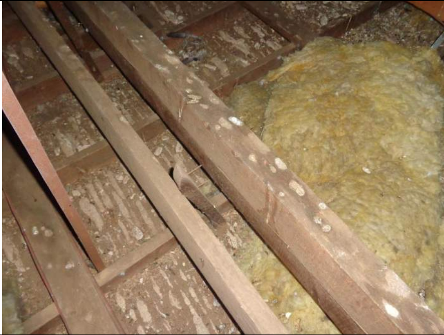
PHOTO 37 – Timber soldier has come away from the hanging beam.
