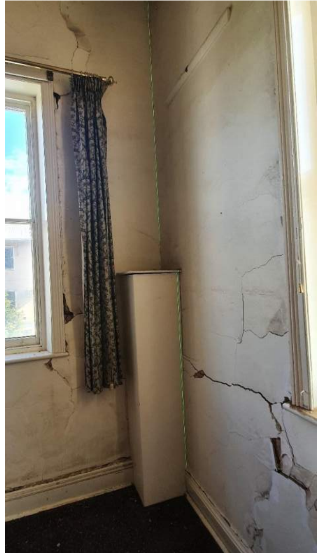
Figure 18 – Cracking to Internal Wall at NW Corner of Western Wing
