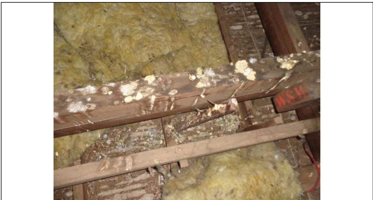
PHOTO 36 – Note the timber soldier has come away from the hanging beam entirely. This has occurred in many locations.
