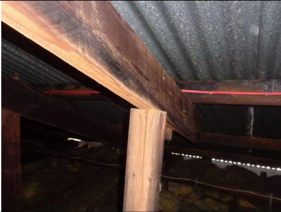
PHOTO 57 – A propped rafter adjacent to a chimney. Very poorly propped and connected.
