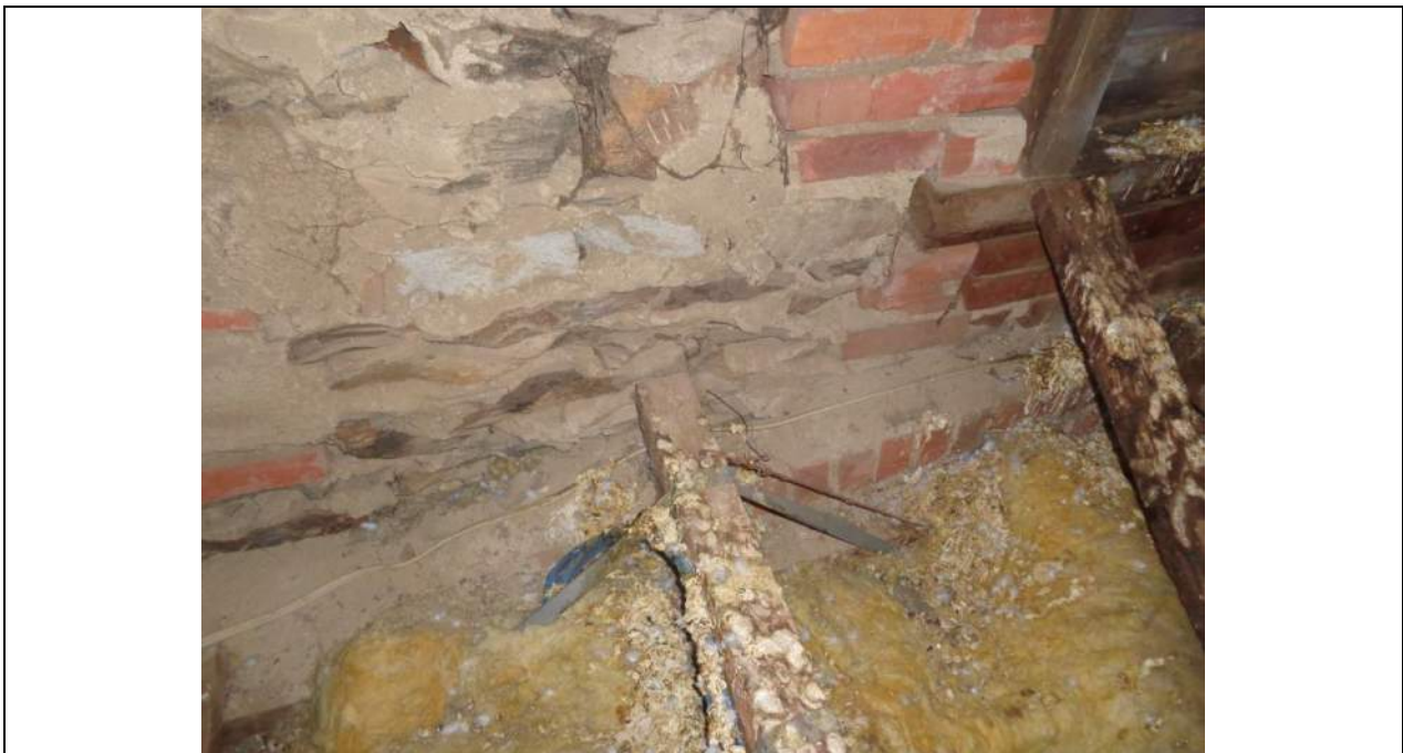
PHOTO 32 – Newer hanging beam supported on a curved brickwork ledge. The timber to the right of the photograph is a prop to the bottom sill of the gable end vent framing.
