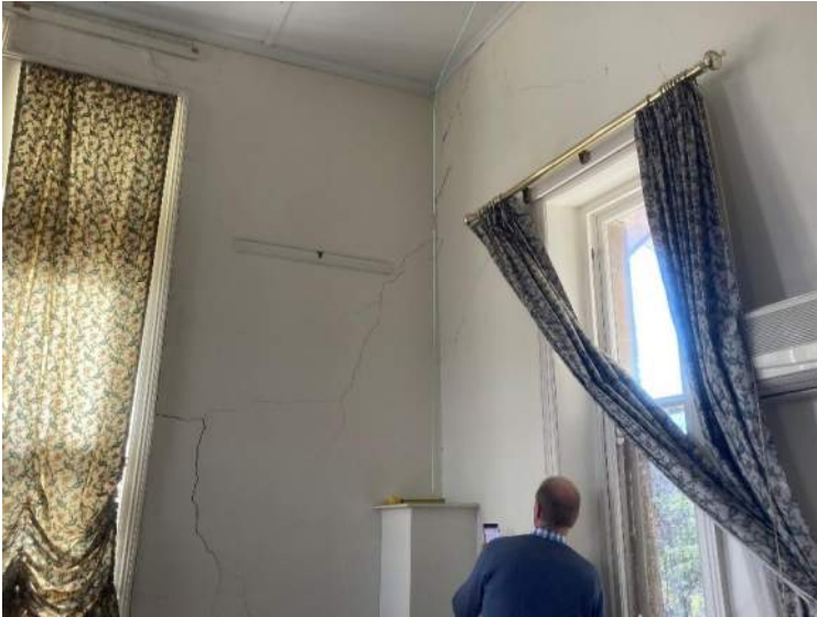
Figure 17 – Cracking to Internal Wall at NE Corner of Western Wing
