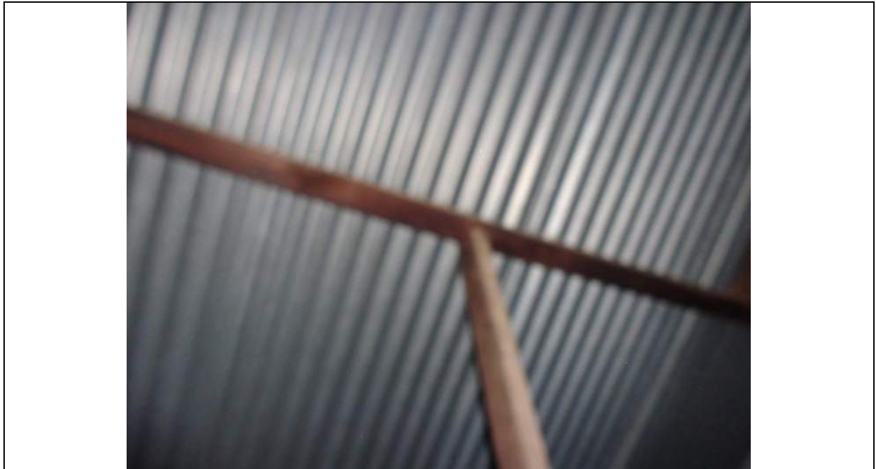
PHOTO 51 – Propping of purlin near the gable end. No tie down or connection apart from skew nailing. (apology for poor photograph quality).
