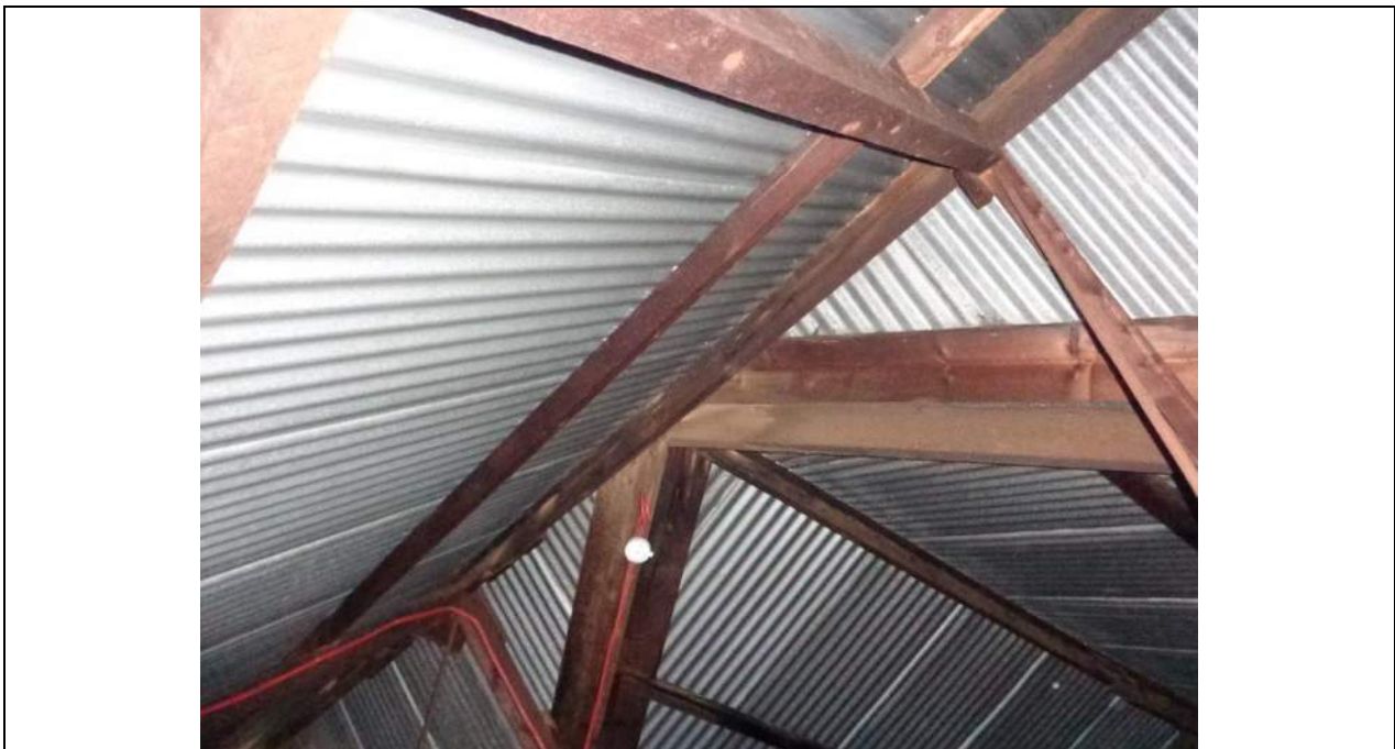
PHOTO 66 – A view of the meeting of the main span and smaller span roof planes to the western end of the roof this time. The valley rafters and ridgebeam seem to extend/cantilever quite a long way and is a potential location of roof sag. The apex point is not well supported at the valley rafter and ridgebeam junction and some additional support would be recommended.
