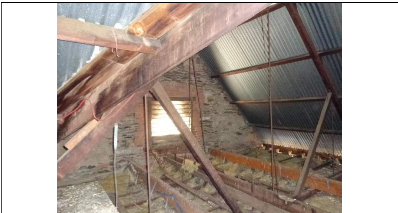
PHOTO 22 – The north facing stonework gable to the eastern end of the roof. The purlins are pocketed into the stonework and some of the stonework is not in good condition with significant mortar deterioration. Some mortar does appear to have been repaired/patched at some stage but generally not around the purlin locations. Two newer rows of hanging beams have been added at some stage.
