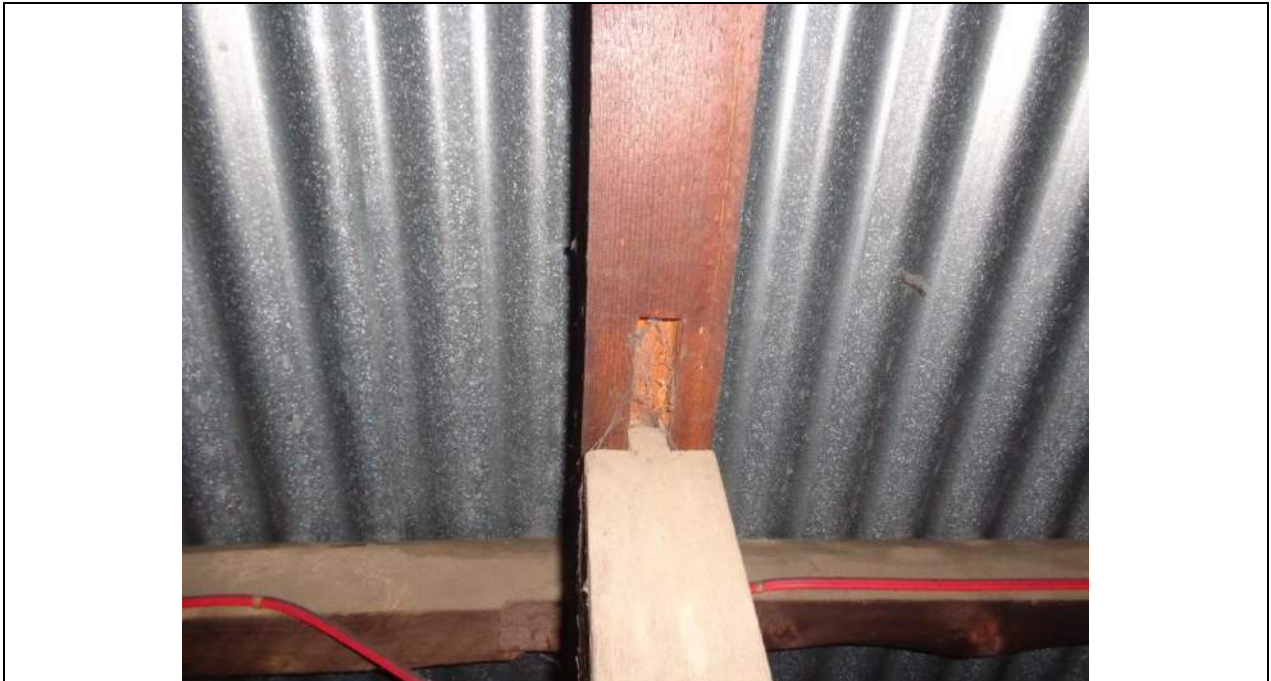
PHOTO 39 – The mortise and tenon joint to the top chord/web location has either slipped, sheared off in part, crushed in part or has become loose/out-of-position because the truss has sagged. A more thorough investigation may be warranted. It is unlikely that the gap is due to poor workmanship.
