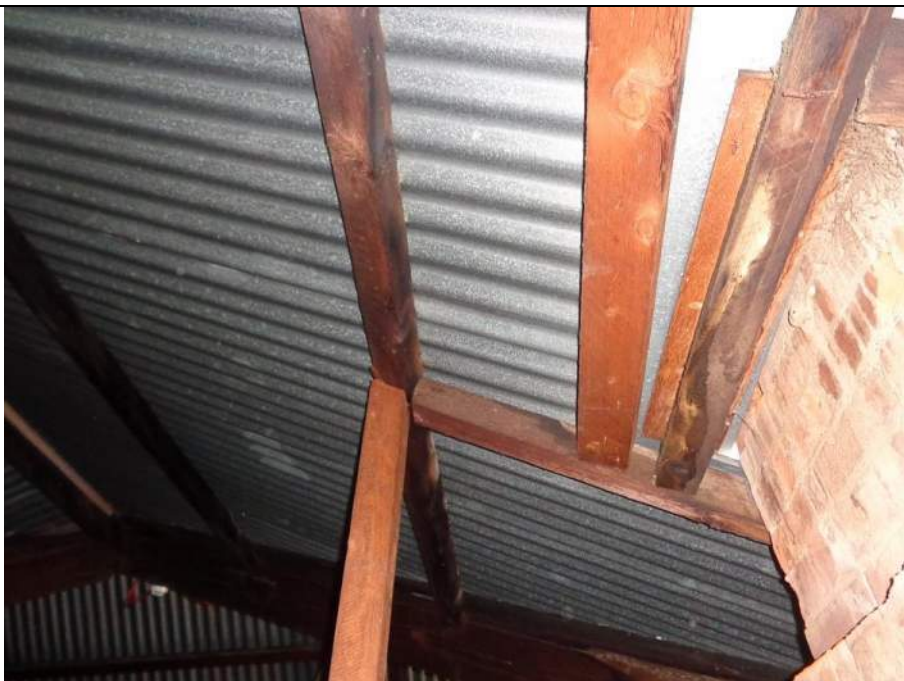
PHOTO 60 – As per photograph 59 showing the propping of the purlin which is carrying additional load due to trimming around a chimney. Most of the trimming looks newer, so it is possible that some trimming work was done when the roof sheeting was replaced last.
