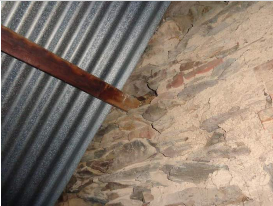
PHOTO 49 – Pocketed purlin not well supported due to localised deterioration around the penetration.
