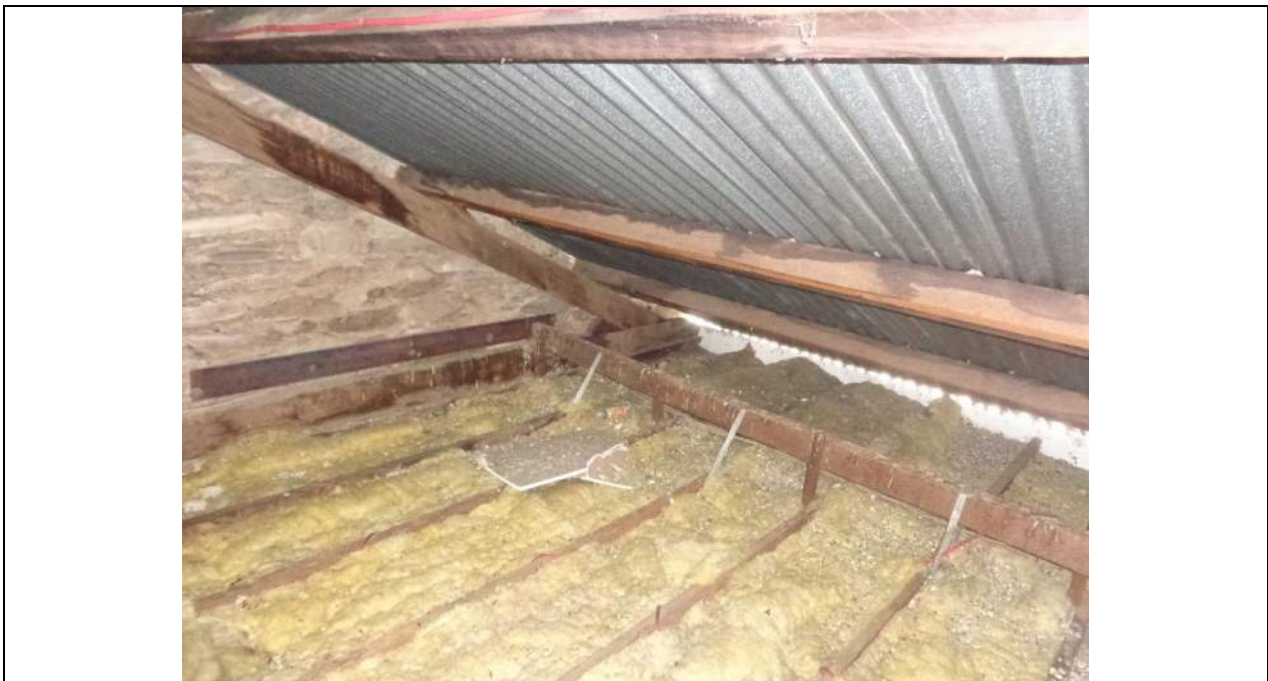
PHOTO 10 – To the east side of the central tower section. The hanging beams and ceiling joists are often over-spanning, excessively deflected or have lost connectivity via a failed soldier member (cleat). The purlins are also exhibiting excessive deflection in many locations. The ceiling is a heavy plaster lathe on timber battens; however, additional ceilings (set down lower) have also been added over time.
