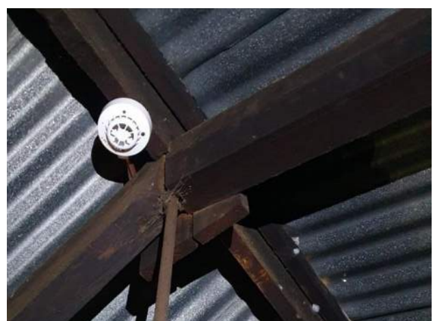
Figure 4 – Separation of Top Chords at Ridge
