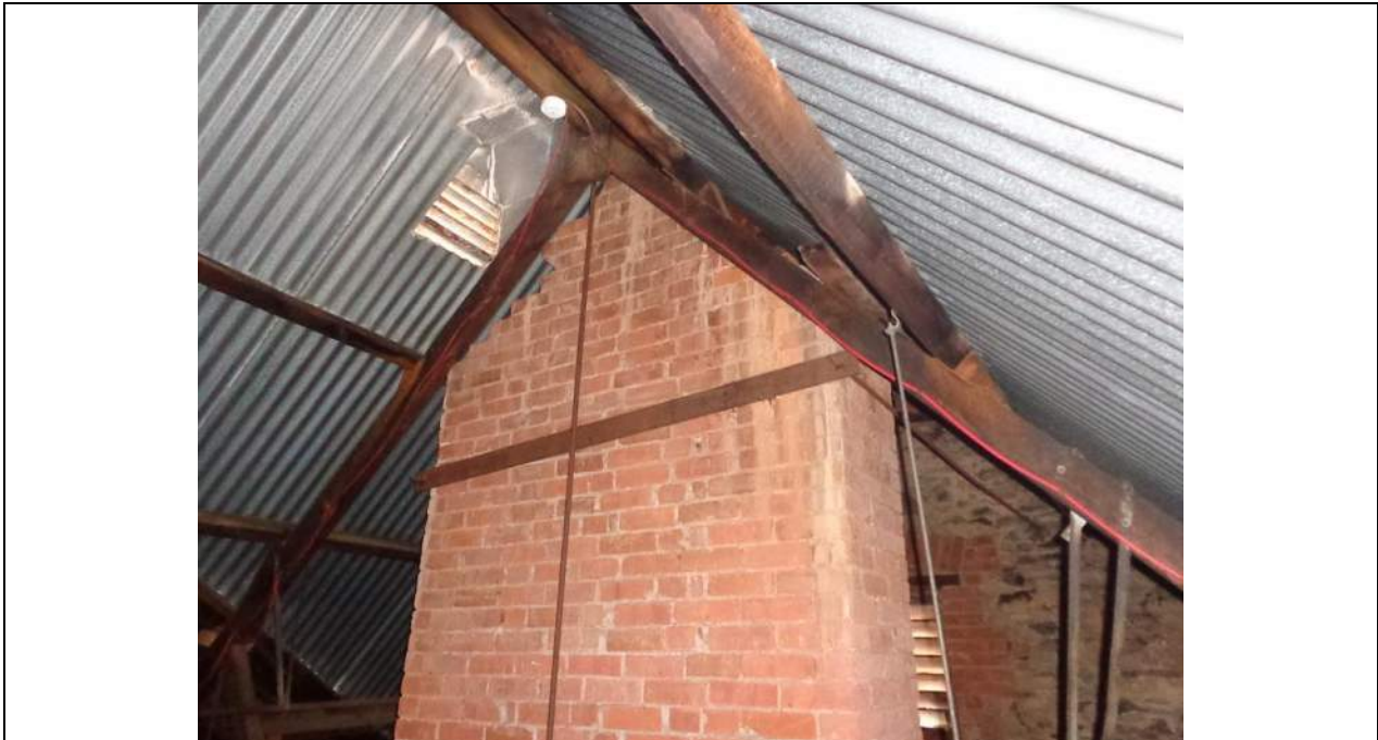
PHOTO 65 – A metal plate and two additional tension tie rods have been added at a higher level for the stone masonry gable end wall and connected around the back of the brick chimney. These were not present to the eastern end although the geometry appears identical.
