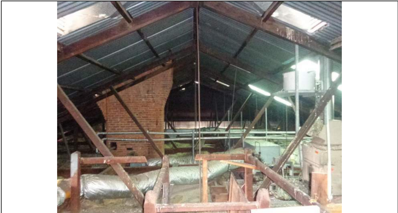
PHOTO 3 – General view of the roof space looking east. Another chimney is evident. There are 8 chimneys in total, 2 to the eastern end, 2 to the western end and 4 to the central section (2 north roof plane and 2 south roof plane). The southern chimneys have been terminated under the roof sheeting. There is significant redundant plant within the roof space.
