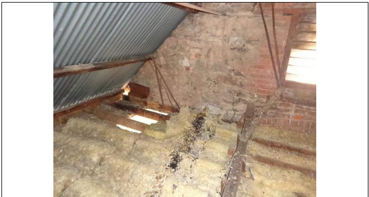
PHOTO 68 – Northern gable to the western end of the roof. The eaves lining is open again allowing easy access for pigeons. The ceiling joists appear to be significantly deflected in this area.
