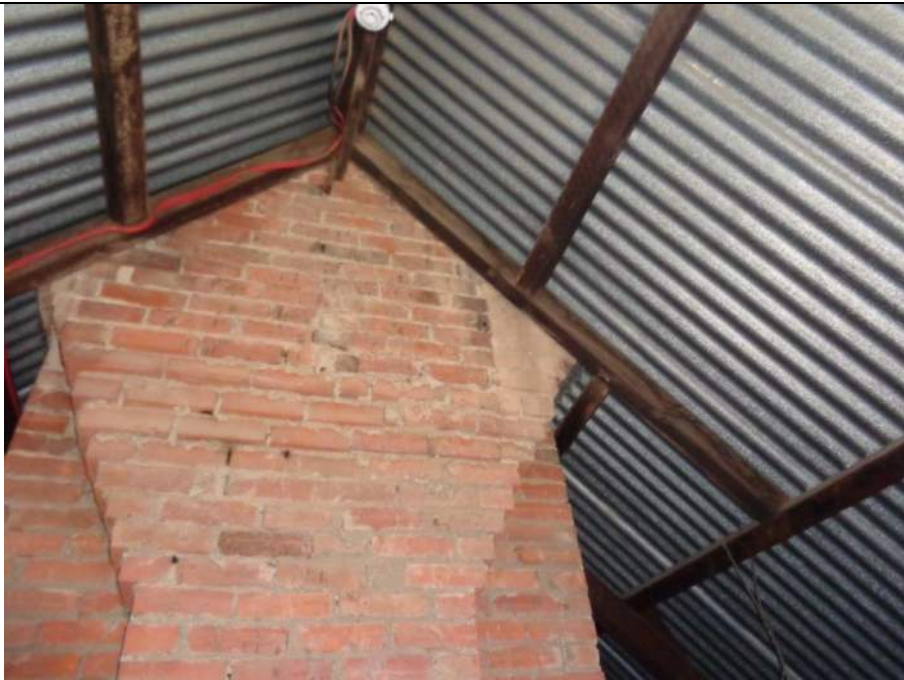
PHOTO 54 – A view of the timber roof framing around the chimney which is less than ideal. The loads should not be transferred to the middle of the purlin as a point load. It was unclear whether the timbers were connected to the chimney or independent of it – the ridgebeam did appear supported; however, a lack of light and height did make some items difficult to confirm.
