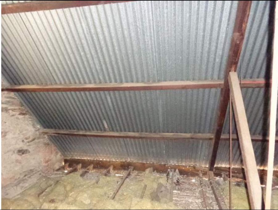
PHOTO 33 – Note the purlin deflection which is quite significant.
