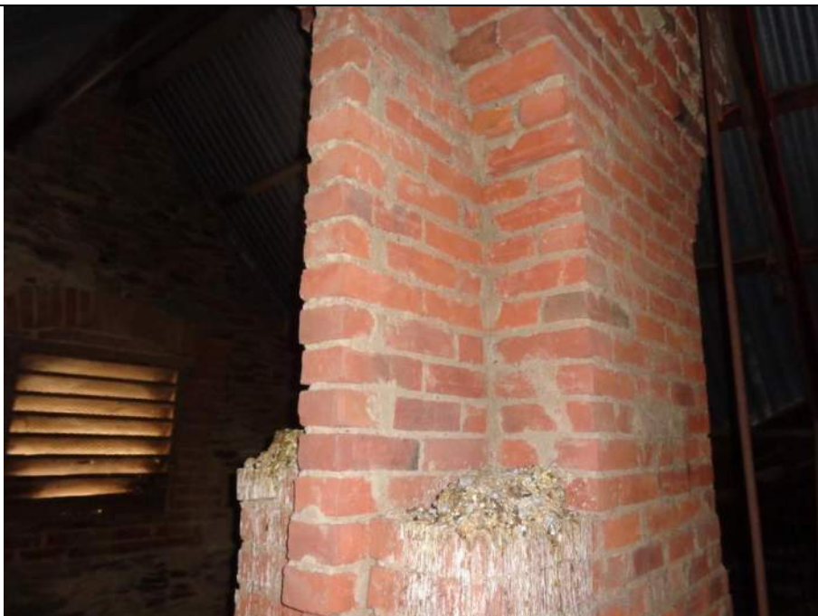
PHOTO 46 – Brick masonry chimney to the southern end of the eastern part of the roof. As mentioned earlier the chimneys will likely need earthquake retro-fitting.
