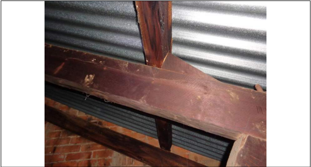
PHOTO 17 – Typical purlin to truss top chord without any specific tie down apart from skew nailing. The purlins span around 3300mm maximum. The split to the truss top chord is a typical drying ‘check’ as mentioned earlier.
