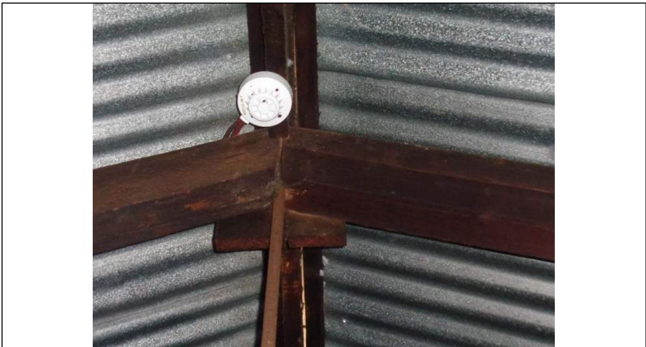
PHOTO 2 – Typical roof truss apex joint with the tension tie rod passing through the two top chords and bolted with a plate on the top face. A gusset board has been applied to one side of the truss top chords predominantly to support the ridgebeam. A number of the gusset boards have split and need attention. Drying splits called ‘checks’ are evident in the top chord to the right at mid depth.
