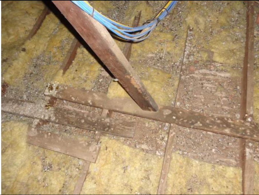
PHOTO 53 – The purlin prop has been placed on a spreader board directly onto the ceiling joists. This is poor practice as the ceiling joists should not be subject to these loads.
