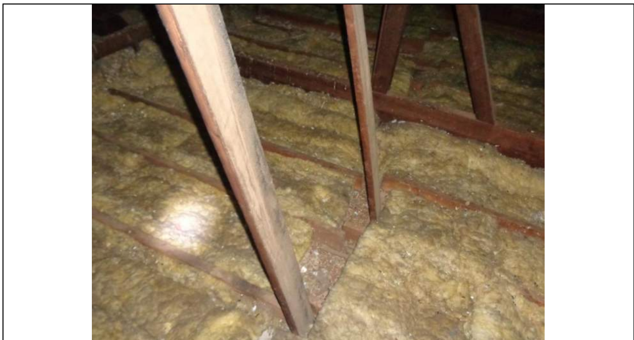
PHOTO 14 – Internal propping of rafters around the chimney locations using narrow timber struts located over the internal load bearing masonry walls. The props are too narrow, are not tied down or effectively fixed. No anti-slip mechanism was provided.
