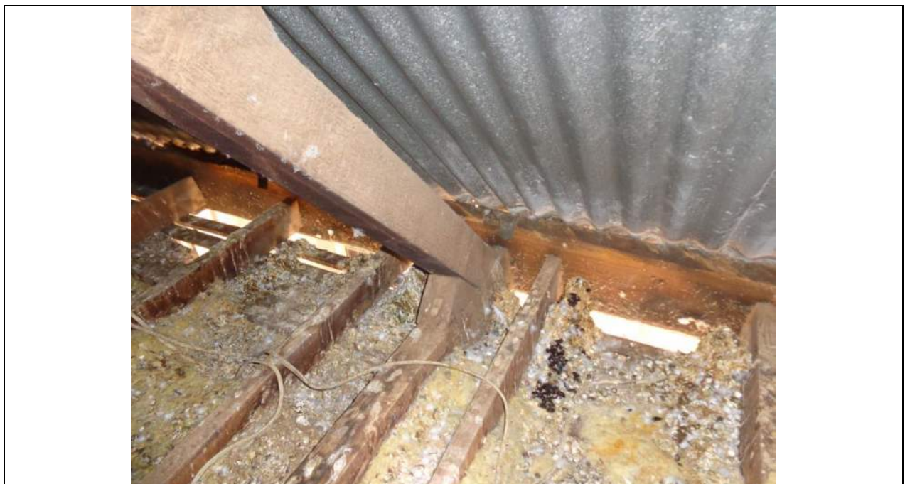
PHOTO 44 – The truss heel joint has a twist in it which is probably not highlighted well on the photograph, but it is concerning. Once again the vented eaves have many pigeon entry points.
