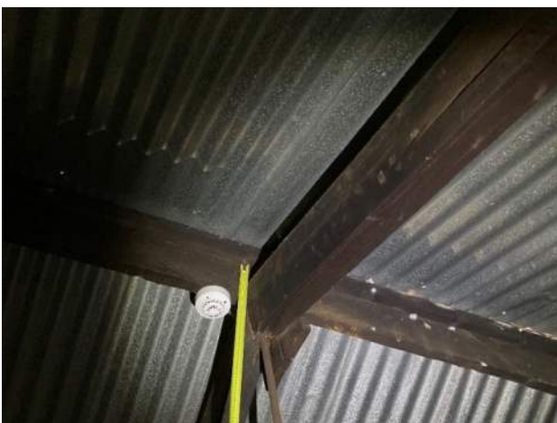
Figure 3 – Split Roof Truss Top Chord
