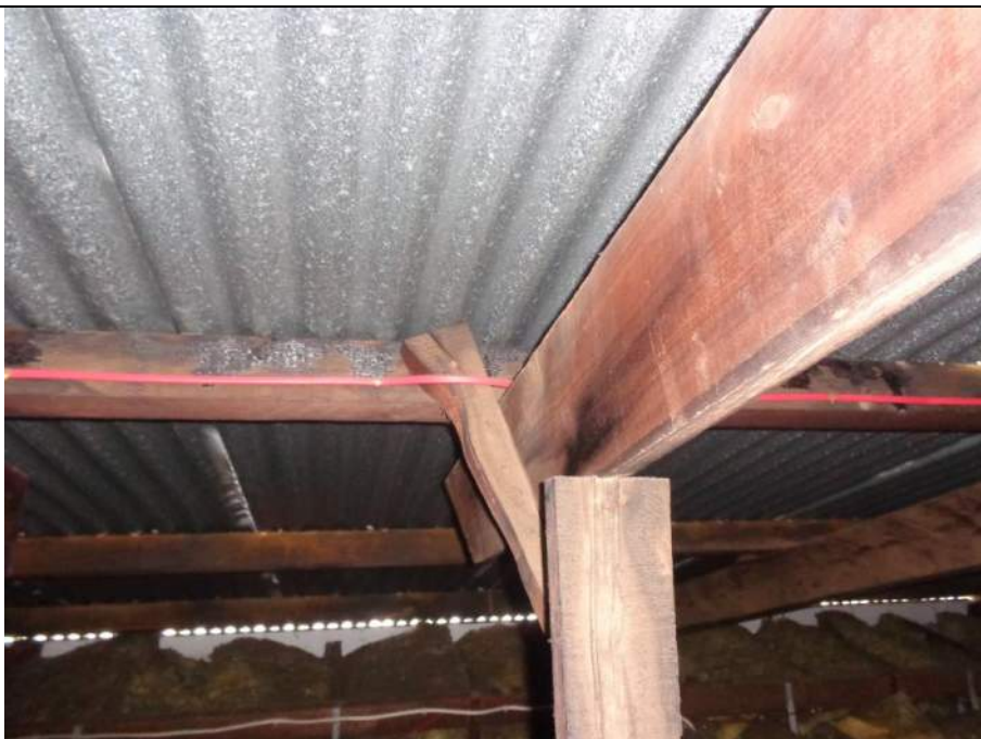
PHOTO 58 – Similar to photograph 57 above. A poorly propped rafter with dubious connection. In addition, the rafter has twisted significantly.
