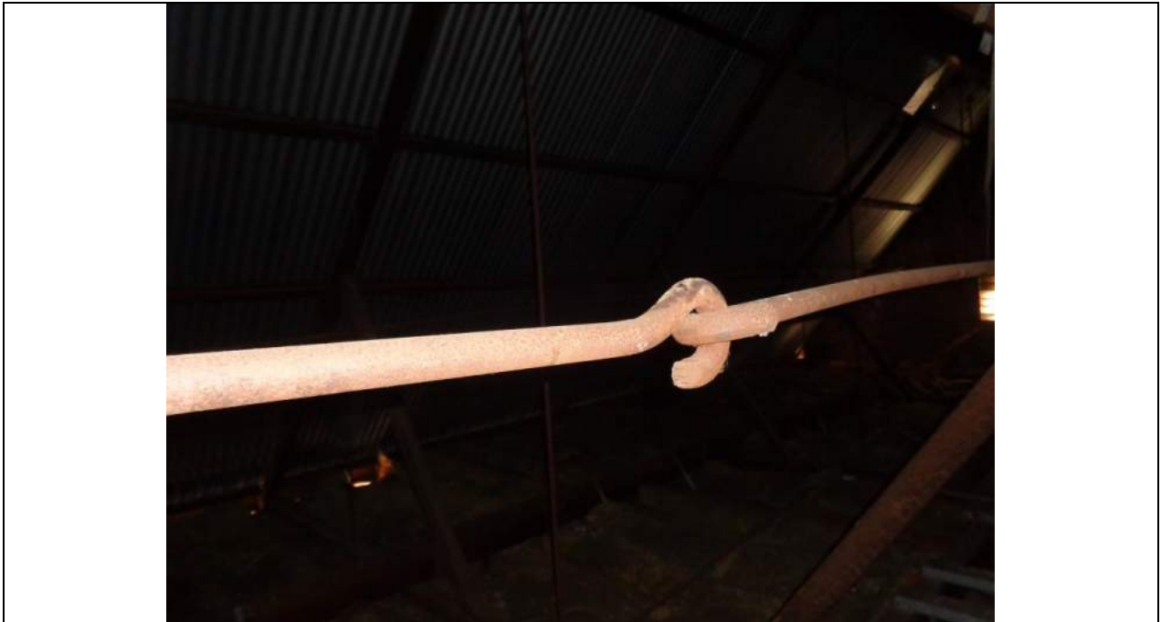
PHOTO 61 – Cast iron tension tie rods to the western gable end of the roof. The tie rods were not present to the eastern end (Why?).
