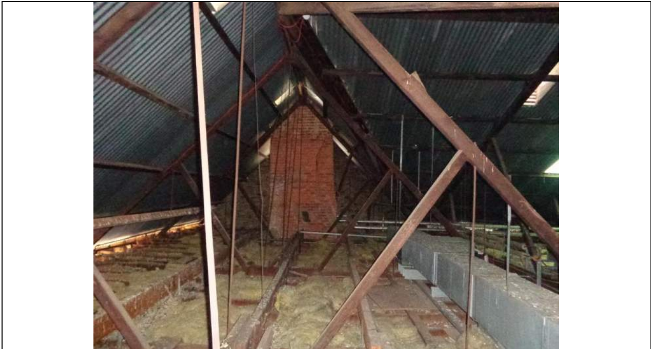
PHOTO 35 – A general view of the eastern end of the roof looking south. Note another substantial brick masonry chimney that will likely need some attention for earthquake purposes. The roof trusses are quite sparse in relation to timber members and quite widely spaced as well with significant ceiling loads applied. It is unclear how the trusses are tied down (if at all) to the supporting walls.
