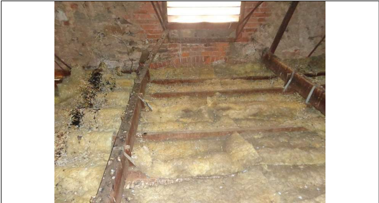
PHOTO 69 – As with photograph 68 above. The ceiling joists appear to be excessively deflected even though the span between hanging beams is not large; however, the deflection may have occurred when there was one central hanging beam which has since been replaced with two.
