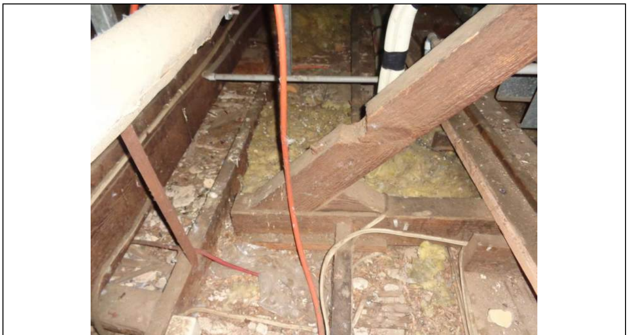
PHOTO 56 – One of the trusses has a significant divert/knot hole taken out of the top chord which is immediately adjacent a large horizontal knot. No cracks or breaks are evident at the location, never-the-less a rectification would be recommended.
