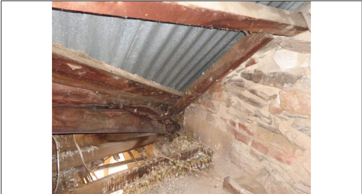
PHOTO 31 – As per photograph 26 but from the opposite side of the hip valley rafter. The valley rafter appears to have some deterioration to the end at the external wall support location. Note the open eaves allowing pigeons to enter -this has occurred in numerous locations.
