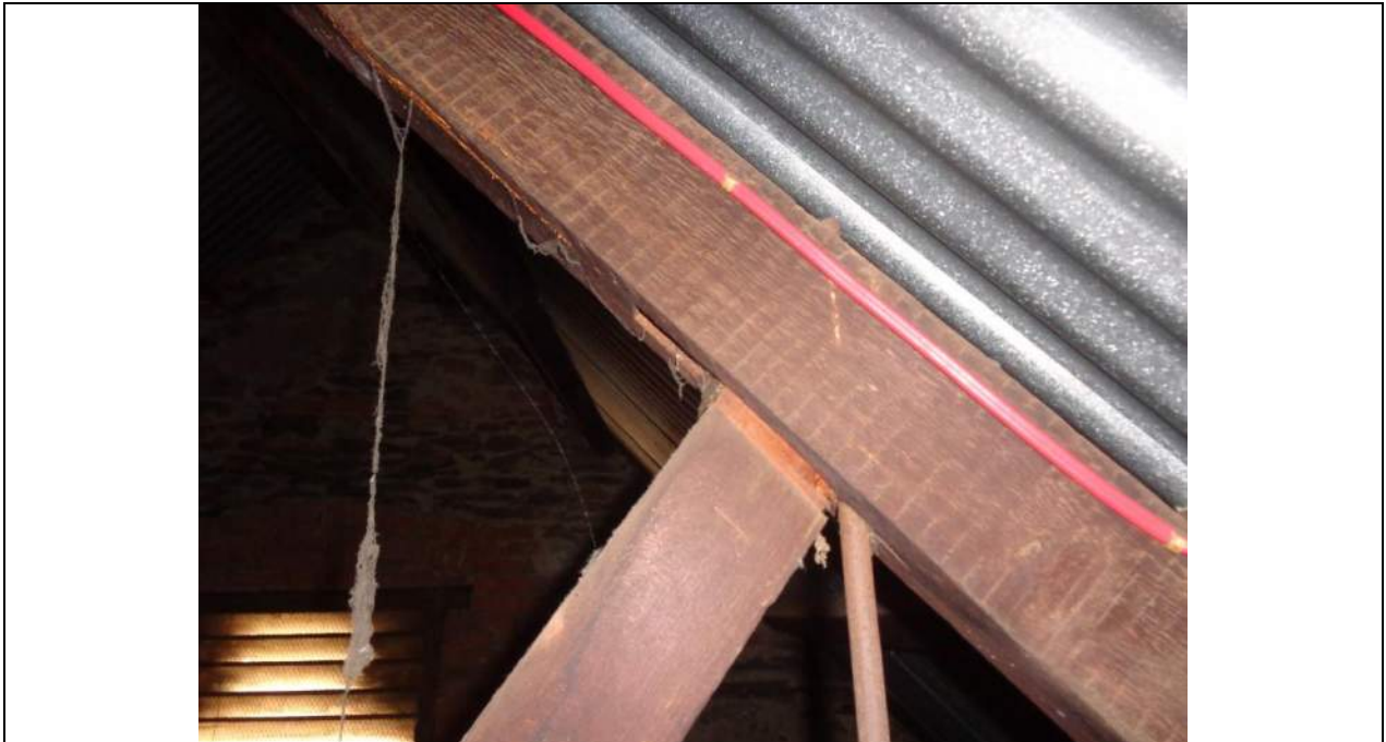
PHOTO 41 – Another slipped top chord/web joint to the eastern end trusses. It appears as if some localised crushing of the tenon might have occurred. The web member has certainly moved significantly out of position.
