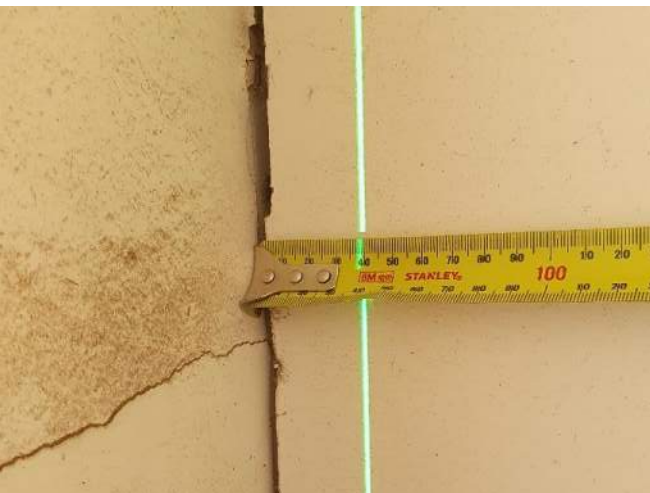
Figure 21 – Bowing of Wall at NW Corner of Western Wing
