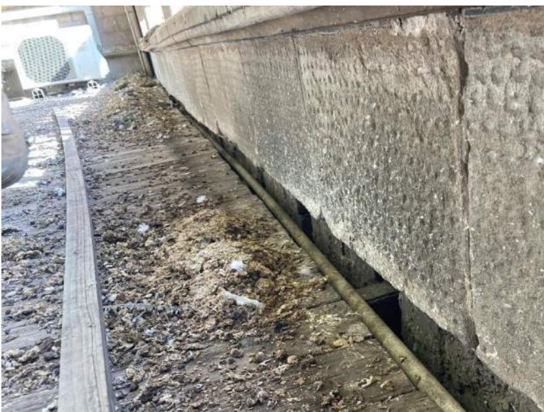
Figure 12 – Separation of Northern Balcony Floor Framing
