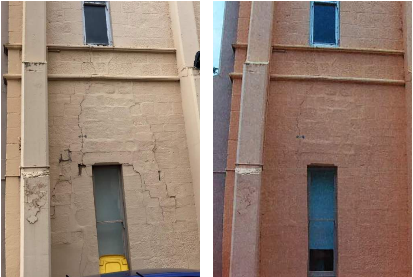
Figure 13 – Comparison of Cracking
