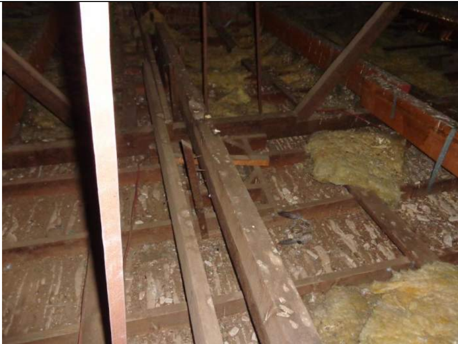
PHOTO 38 – More timber soldiers have come away from the hanging beam.
