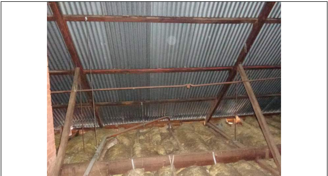
PHOTO 62 – Another view of the tension tie rods which extend from stone masonry gable northern end to stone masonry gable southern end. The tie rods are quite heavy and are being supported from the truss top chords at a few locations.
