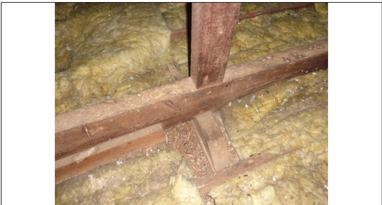
PHOTO 8 – As per photograph 7 above showing the vertical web member aligning over the internal wall support. Any wall changes that may occur as a result of the refurbishment works may have to take into consideration some roof loads being applied to internal walls rather than wholly external walls.
