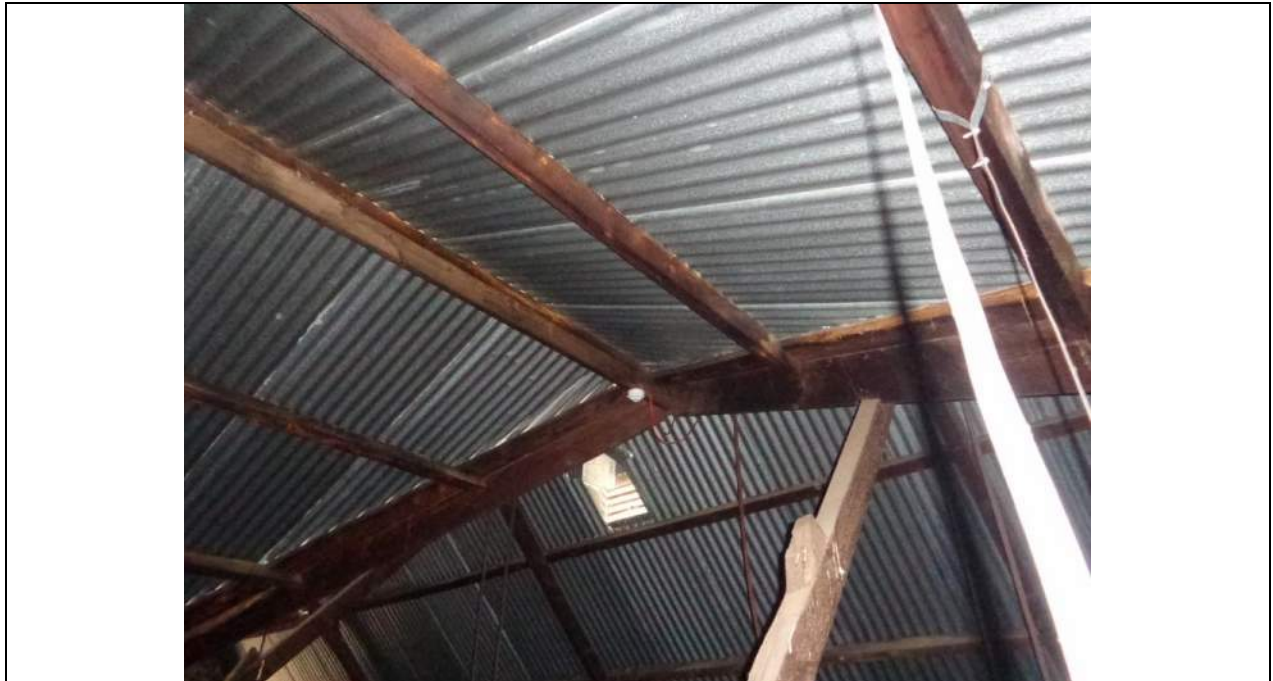
PHOTO 55 – A view of the junction of the main roof (25-degree pitch) with the perpendicular roof (45-degree pitch). The apex point is not well supported at the valley rafter and ridgebeam junction. For such a large span roof, minimal timber has been adopted. Some water damage is evident along the valley members and purlin ends.
