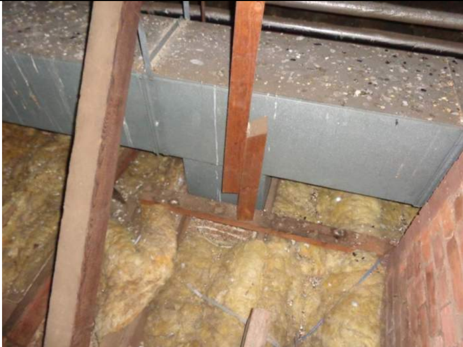
PHOTO 59 – Rather poorly done propping of purlin member. The propping doesn't appear to be original build.
