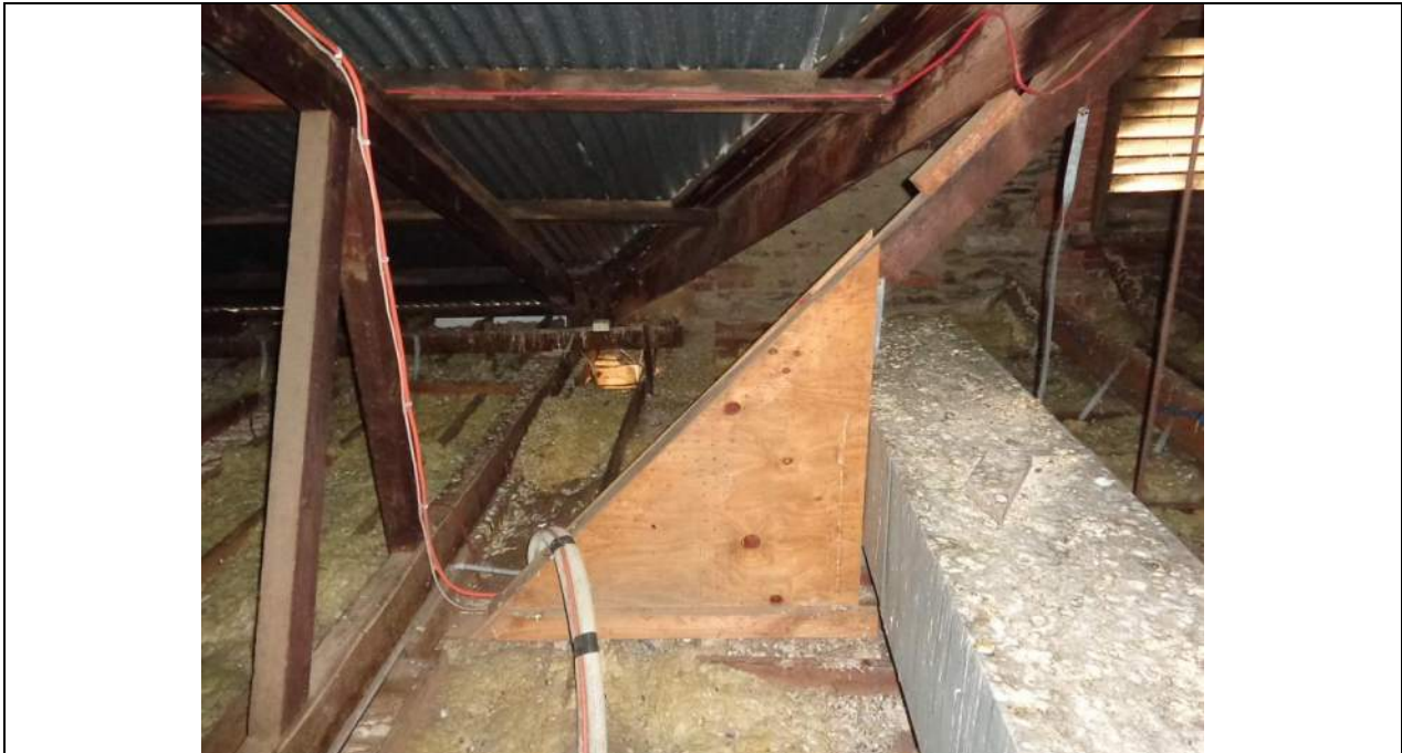
PHOTO 19 – To the eastern end of the building the main span trusses finish and smaller span trusses at right angles form the gable ends of the roof with some conventional hip valley rafters incorporated. The smaller span trusses are at almost 45-degree pitch and have minimal top chord restraint to the internal wall end. One of the trusses has had a plywood gusset repair at some stage, the reason was not obvious.
