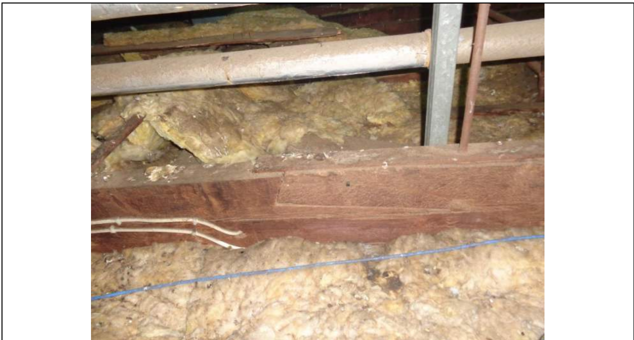
PHOTO 70 – Another view of the bottom chord splice detail to the main span truss. The splice detail did not seem to be consistently in the same location.
