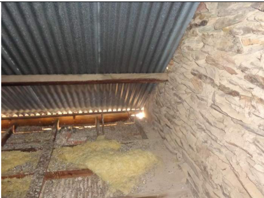
PHOTO 50 – The fascia beam to the background has rotted out and left a significant gap.
