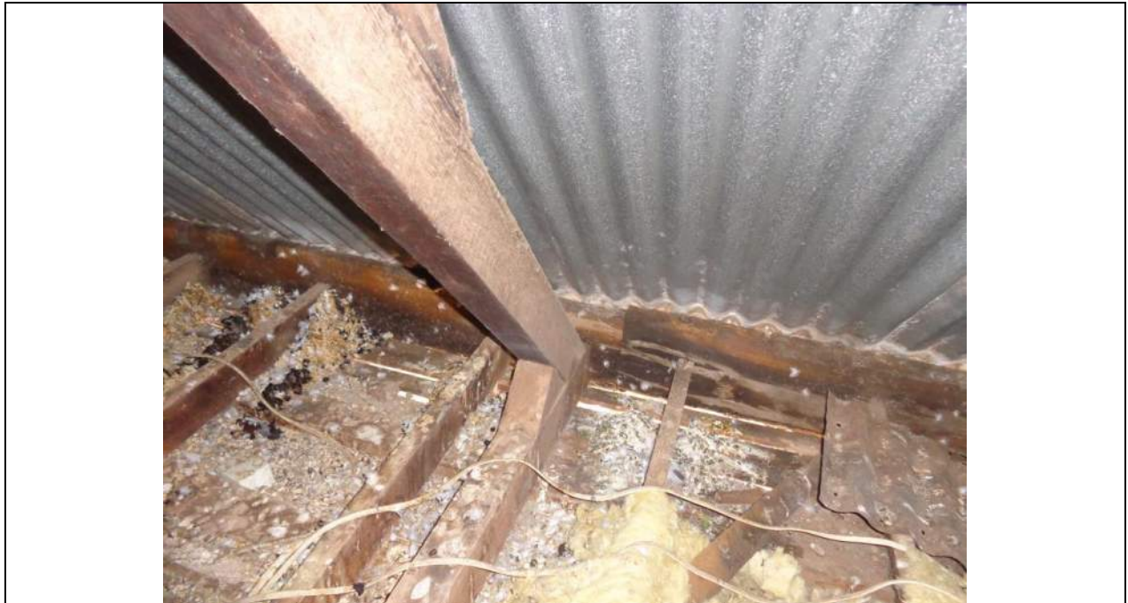
PHOTO 43 – The eastern most external wall. The fascia beams are showing some water damage and deterioration. A number of the trusses have twisted at the heel joint which is concerning. It is not evident that the trusses have any tie down to the external wall, it may be the weight of the heavy ceiling that has combatted the uplift potential over the years.
