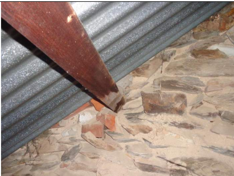
PHOTO 30 – The mortar has deteriorated and the support for the purlin doesn't appear robust.
