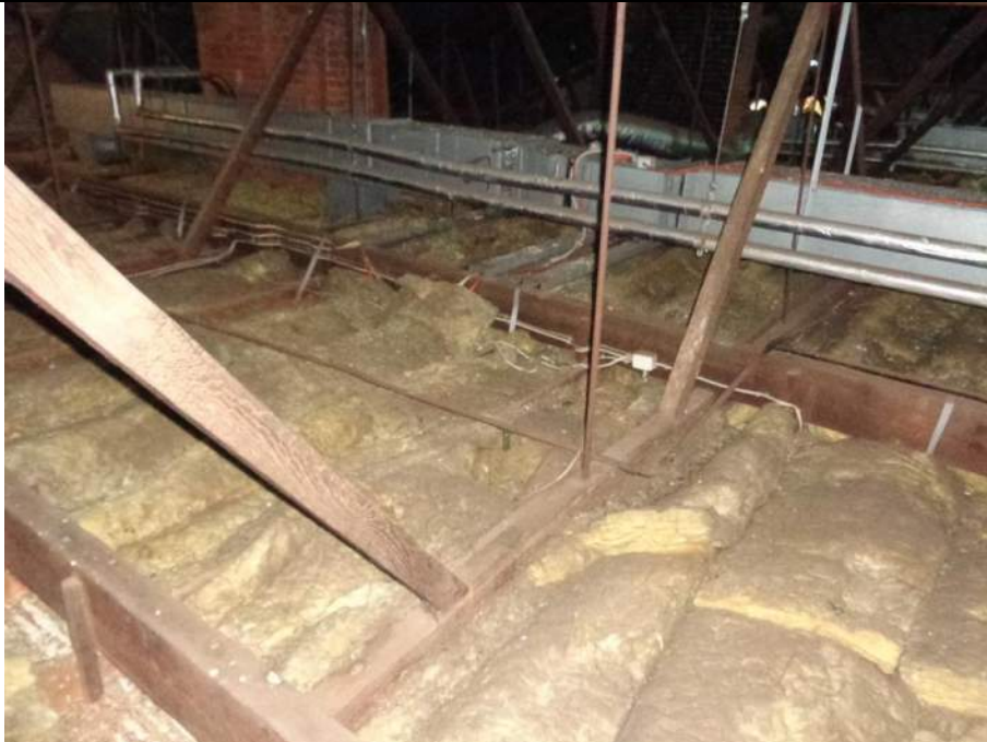
PHOTO 63 – A view of the smaller span trusses this time to the western end of the roof. Note this time there is no central hanging beam but two newer hanging beams at third points to the trusses. Metal straps have been added to support the ceiling joists.
