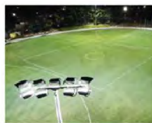
03 Sport and Field Lighting Oval Lighting and Tennis Court lighting suitable for training and games
