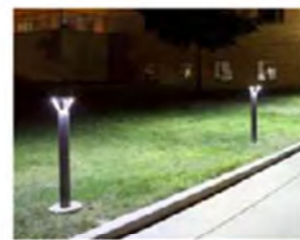
04 Bollard & Area Lighting Bollard lighting to less trafficked primary and secondary pathways.
