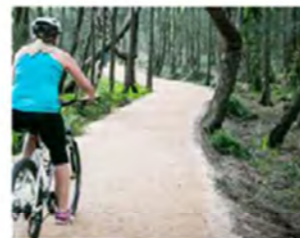
02 Tertiary Paths Compacted rubble for ancillary paths suitable for bike riding, as well as loose gravel paths for informal pathways
